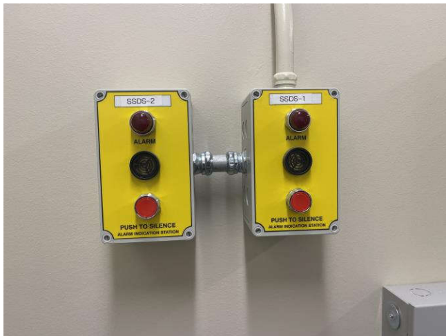
Photo 3: View of the AIS in Custodian's Office.
