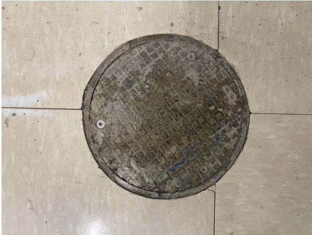
Photo 7: View of SSDS monitoring point in school lobby.
