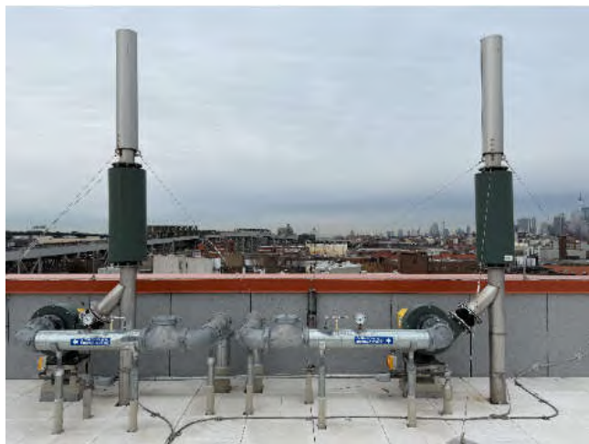
Photo 5: View of both roof-mounted SSDS fan units.
