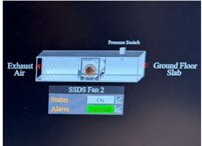
Photo 2: View of the BMS associated with SSDS-2.
