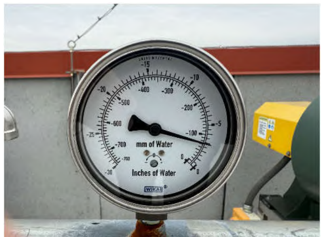
Photo 6: View of the typical SSDS fan vacuum gauge.
