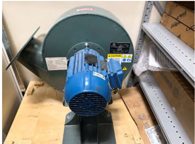
Photo 4: View of spare SSDS fan unit in Room 306.
