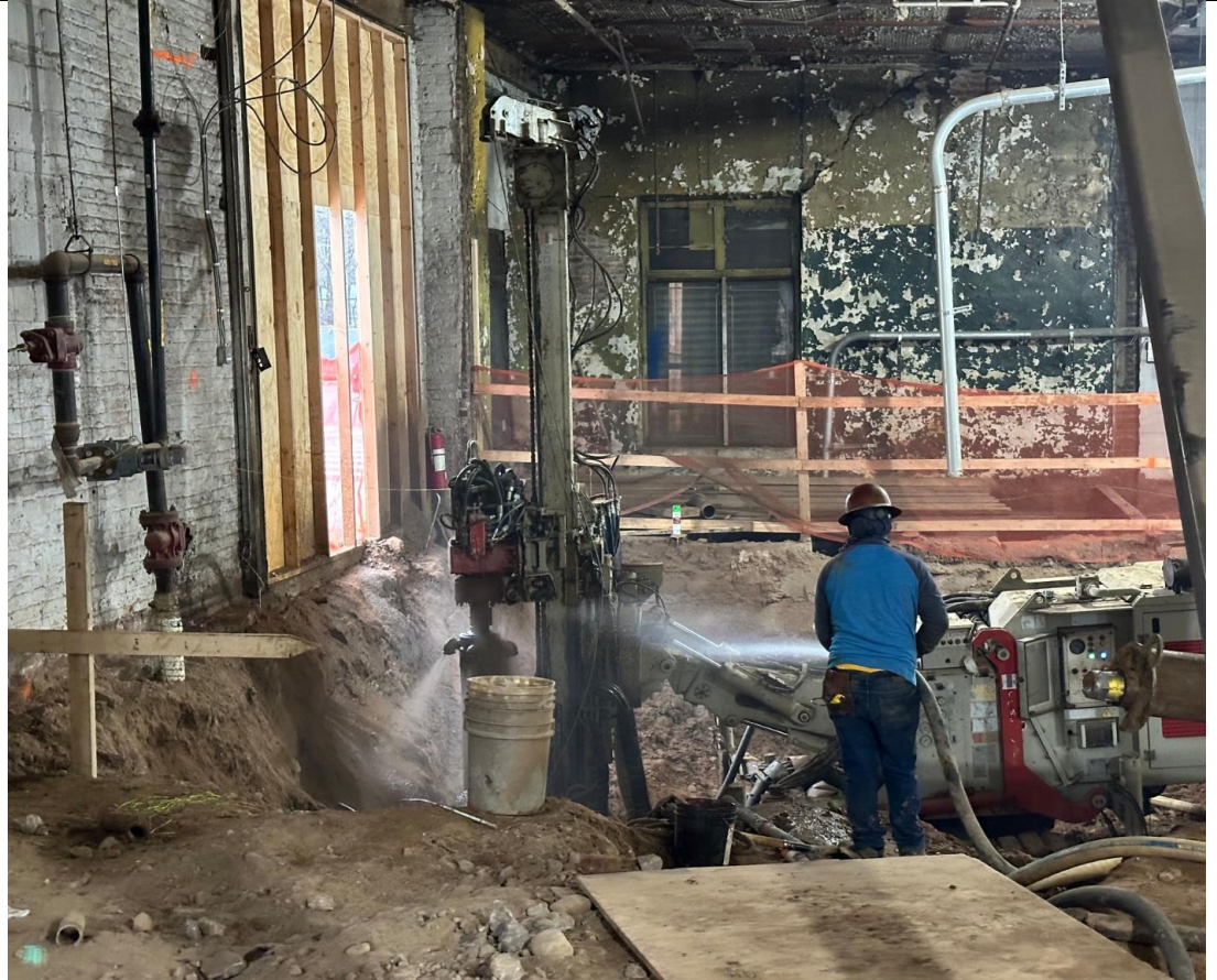
Photo 2 – View of the use of water as dust suppression during support of excavation pile installation.
