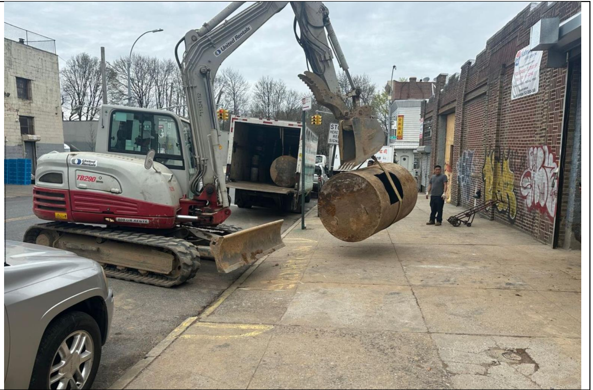
Photo 3 – View of loading tanks for off-site disposal.
