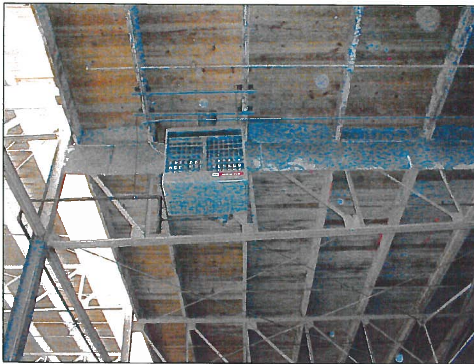
View of the heating system throughout the warehouse
