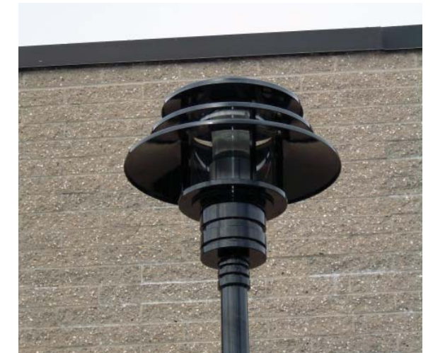
FIGURE 6-9B: VIEW OF THE CANDELA FIXTURE
