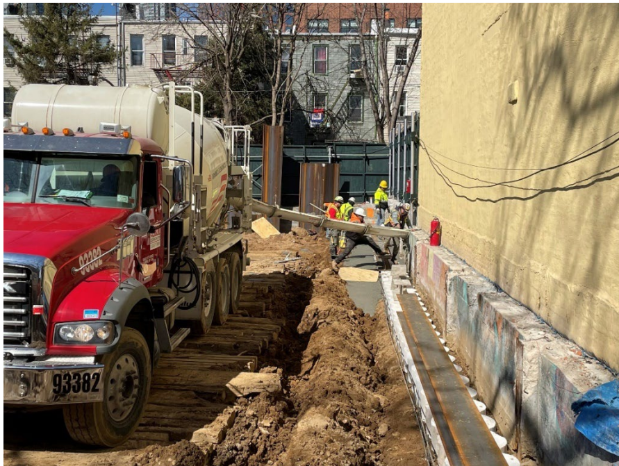
Photo 2: View of concrete pour for eastern soil mix wall installation facing north.
