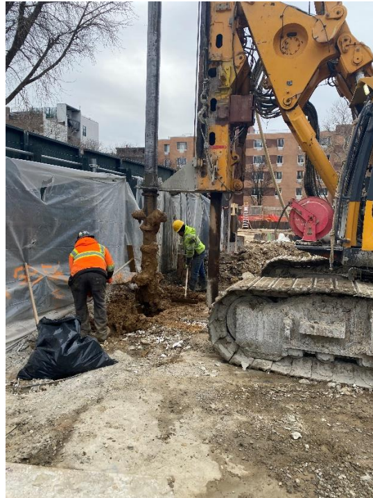
Photo 1: View of soil mix wall installation along the northeastern perimeter of the site.
