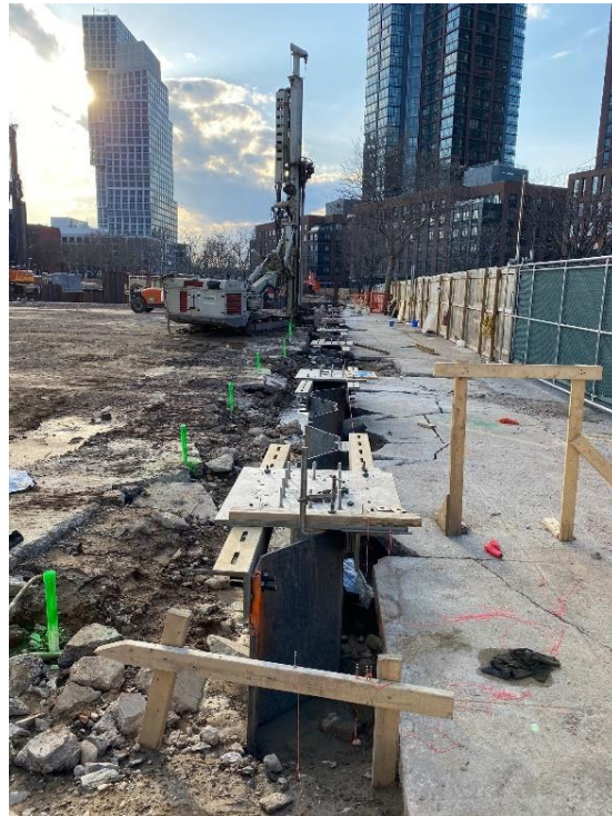
Photo 1: View of tent anchor & dewatering posts installation along the northern portion of the site.
