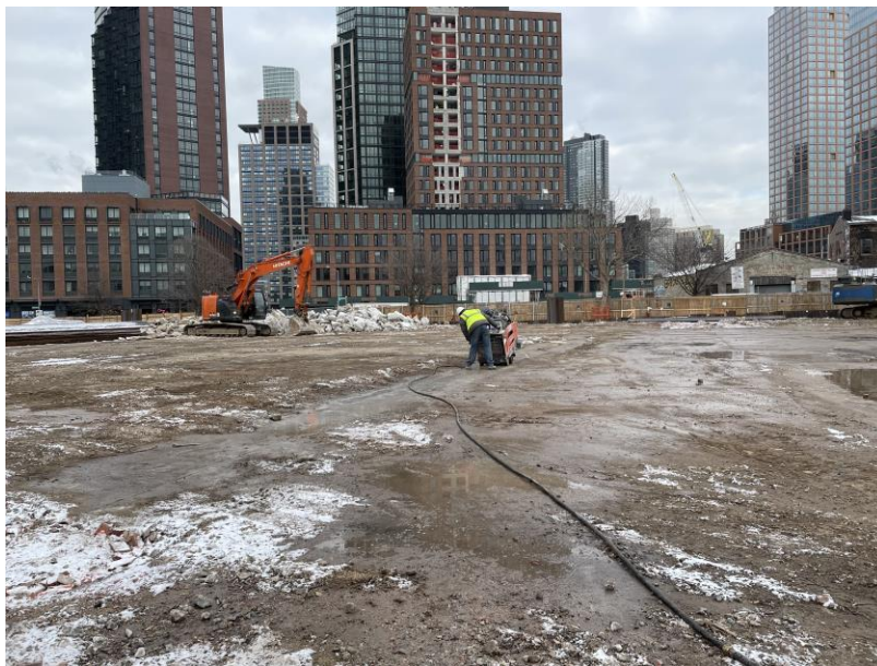
Photo 2: View of contractor saw cutting concrete to prepare for sheet pile wall installation.
