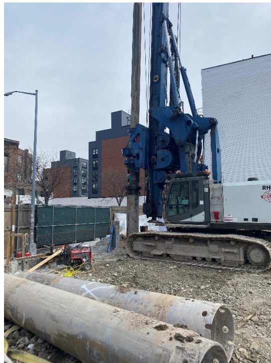
Photo 2: Alternate view of soil mix wall installation along the northeastern perimeter of the site.
