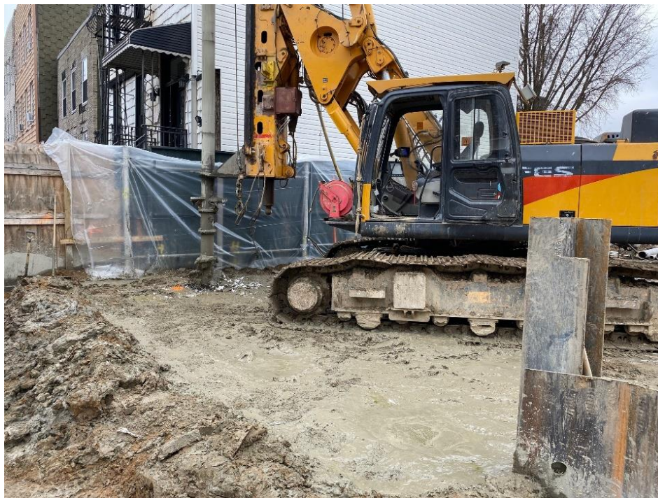
Photo 2: View of soil mix wall installation at northeastern perimeter of the site.
