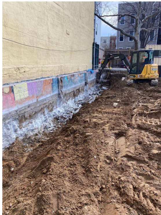
Photo 2: View of preparation for installation of soil mix wall along eastern perimeter of the site.
