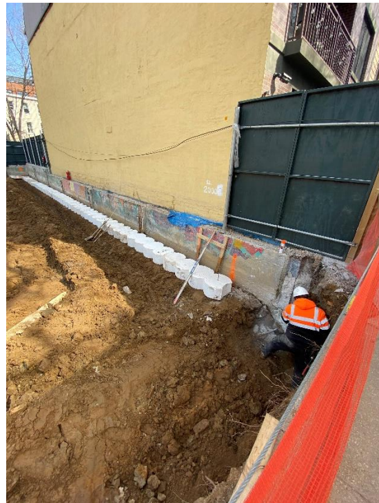
Photo 2: View of formwork installation for soil mix wall on eastern portion of site.
