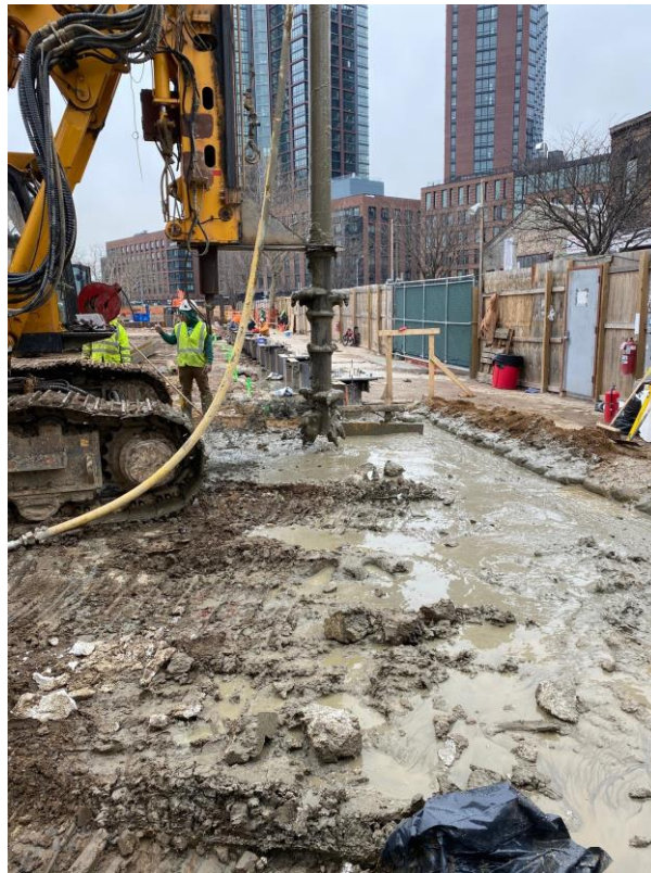
Photo 2: View of soil mix wall installation along northeastern perimeter of the site.
