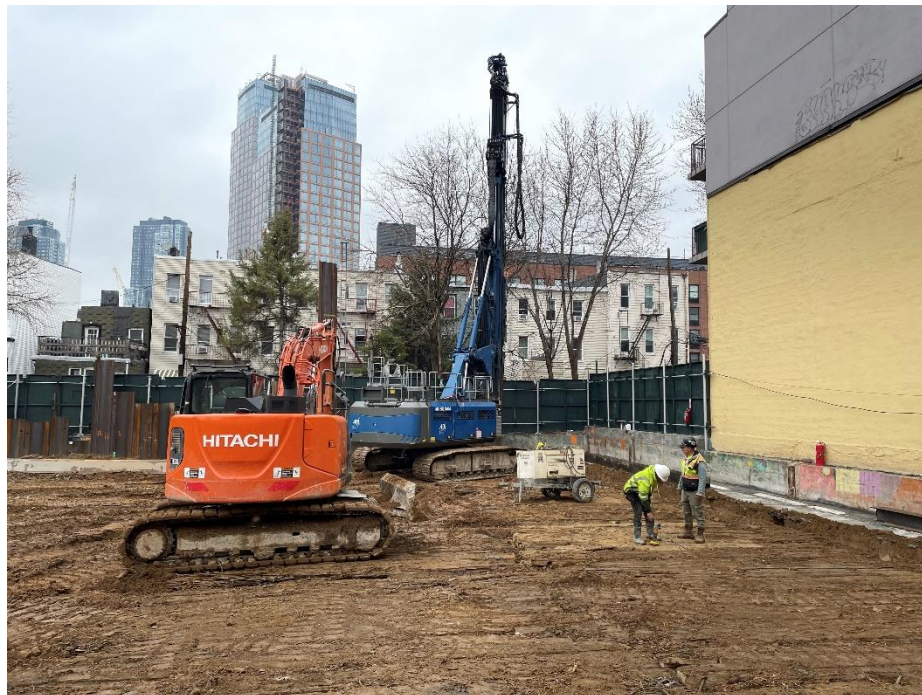
Photo 2: View of preparation for soil mix wall installation in Lot 57 facing north.
