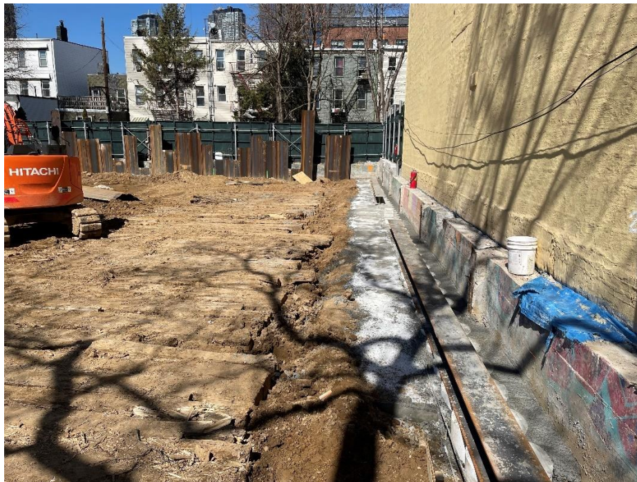
Photo 2: View of formwork for soil mix wall installation on Lot 57 facing north.
