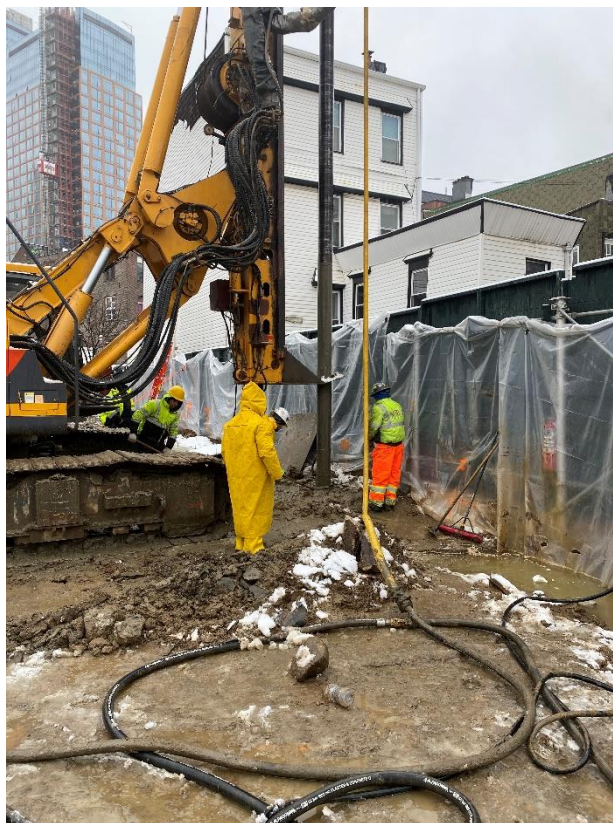
Photo 2: Alternate view of soil mix wall installation along the northeastern perimeter of the site.
