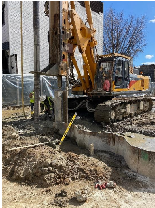
Photo 2: View of soil mix wall installation along northeastern perimeter of the site.
