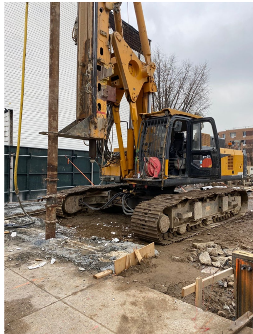
Photo 2: View of installation of soil mix wall at northeastern perimeter of the site.
