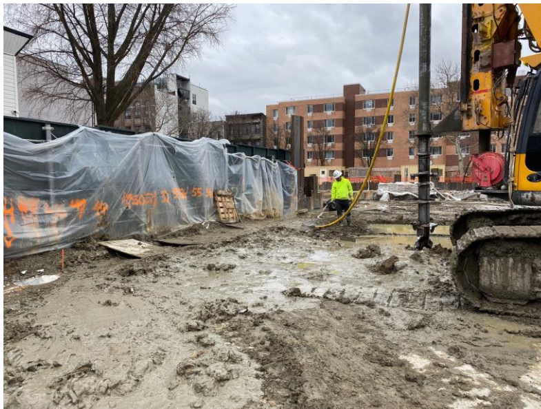
Photo 2: View of soil mix wall installation along the northeastern perimeter of the site.
