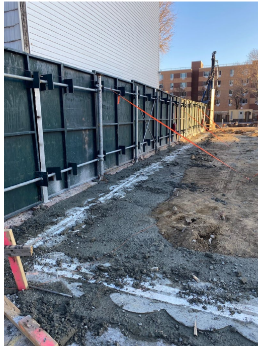
Photo 2: View of styrofoam formwork and concrete pour in preparation for OU-1 soil mix wall.
