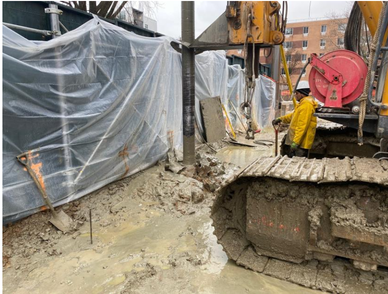
Photo 1: View of soil mix wall installation along the northeastern perimeter of the site.
