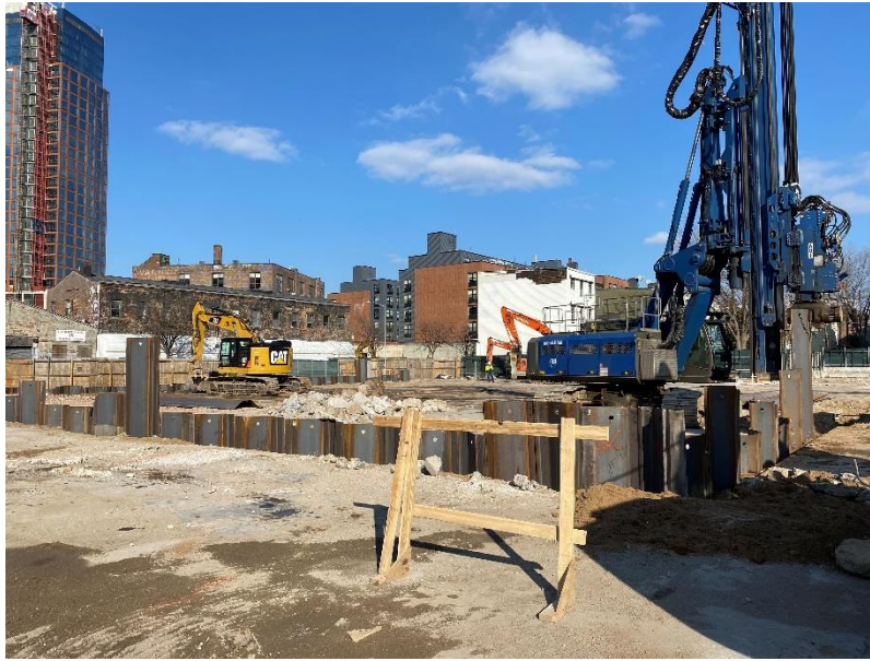
Photo 1: View of contractor installing sheet pile wall along the western portion of the Site.
