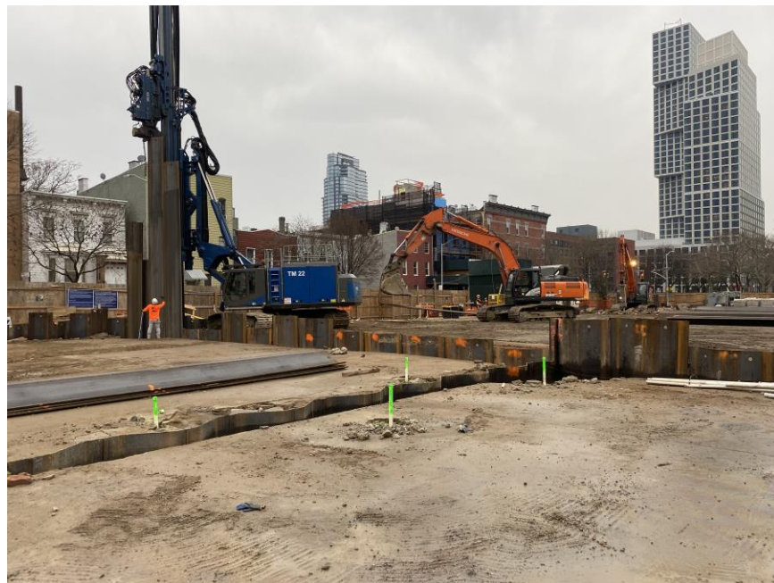
Photo 2: View of sheet pile wall installation on the boundary of NuHart East and NuHart West.
