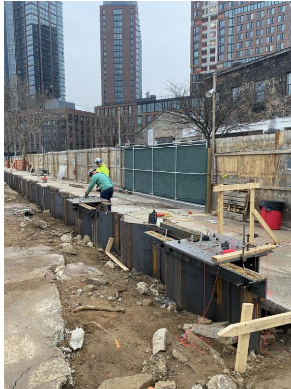
Photo 1: View of tent anchor installation along the northern portion of the site.
