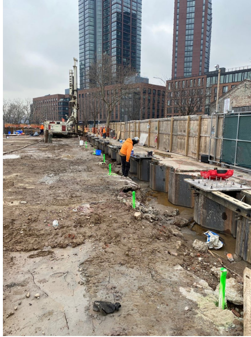
Photo 1: View of tent anchor & dewatering posts installation along the northern portion of the site.
