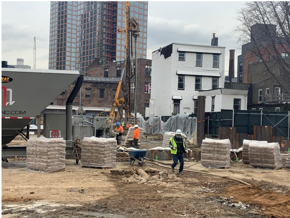
Photo 2: View of the contractor preparing grout for soil mix wall, facing northeast.
