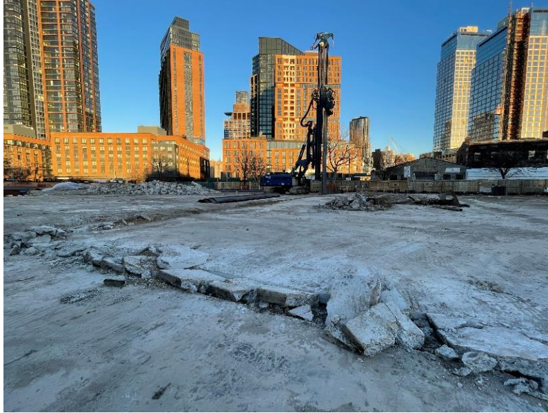
Photo 1: View of contractor installing sheet pile wall along the western portion of the Site.
