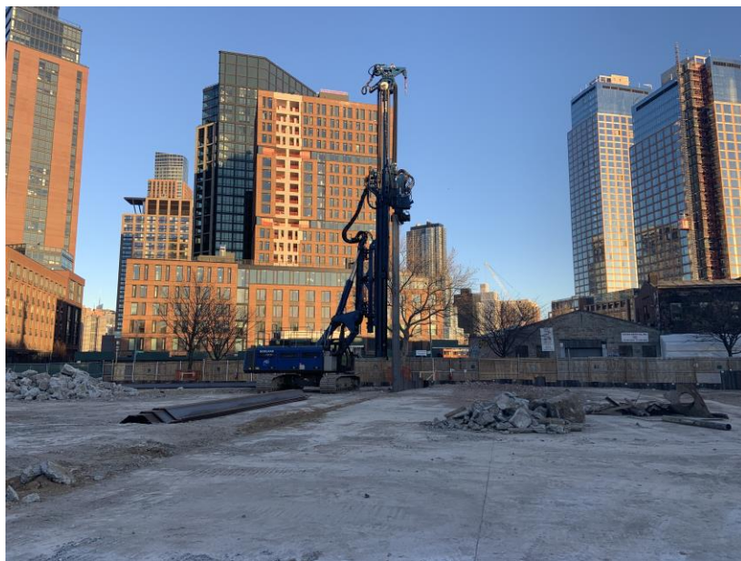
Photo 2: View of contractor installing sheet pile wall on the western portion of the site.
