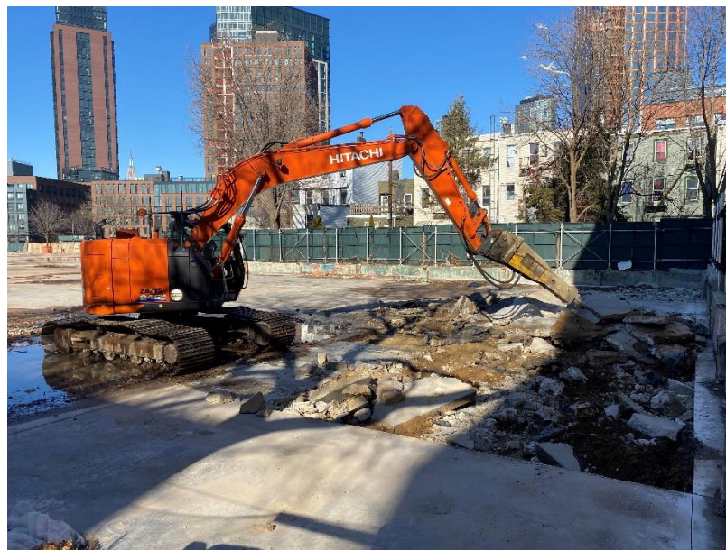
Photo 2: Alternate view of contractor preparing the area for the soil mix wall.
