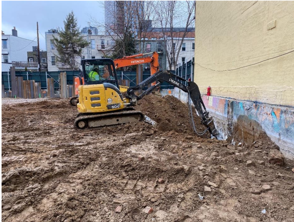
Photo 1: View of preparation for soil mix wall installation at eastern perimeter of the site.
