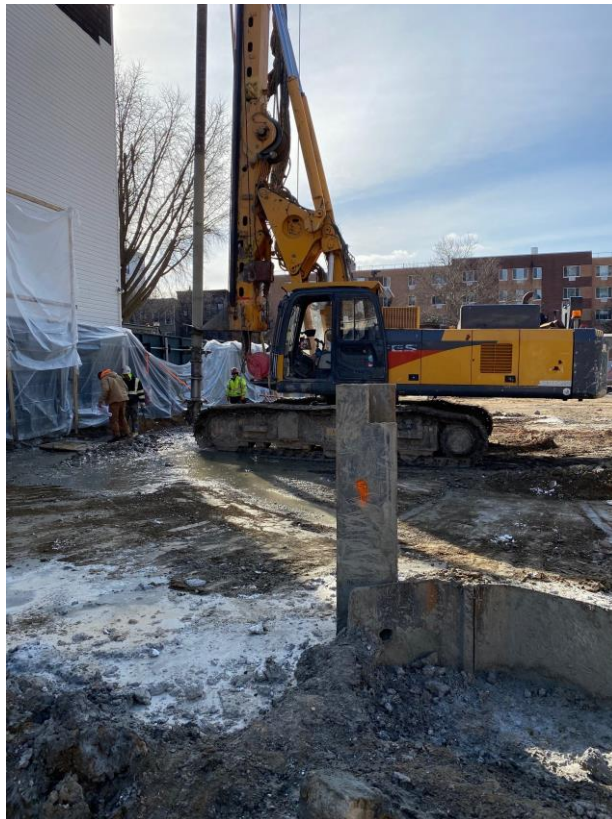
Photo 2: Alternate view of soil mix wall installation along the northeastern perimeter of the site.
