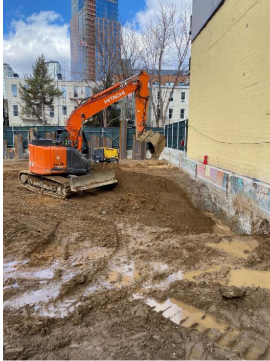
Photo 1: View of preparation for soil mix wall installation along eastern perimeter of the site.
