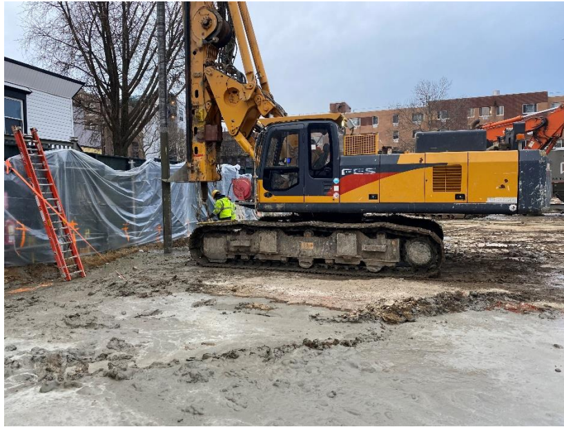
Photo 1: View of soil mix wall installation along the northeastern perimeter of the site.
