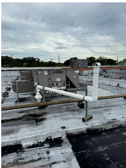
Photo #1 – View of rooftop SSDS fan in operation.
