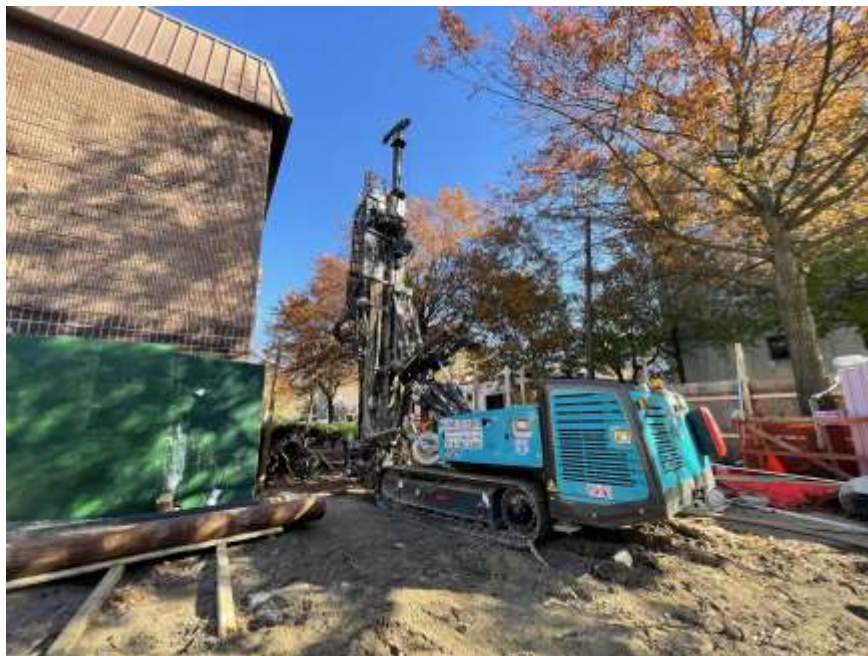
Photo 2: View of Anel installing soldier piles in the southeastern part of the site (facing southeast).
