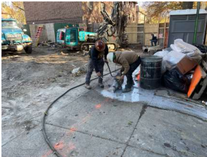
Photo 2: View of Rise applying water to the concrete sawing activities to minimize dust (facing east).
