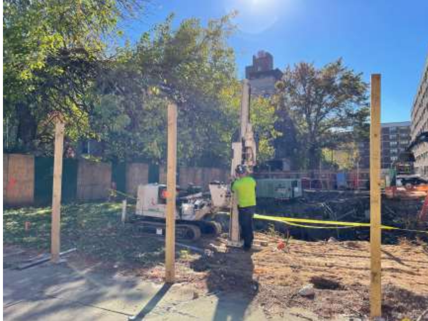
Photo 1: View of Lakewood advancing a soil boring in the southwestern part of the site (facing northwest).
