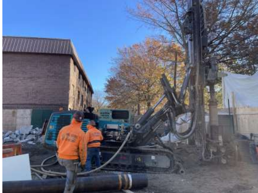
Photo 1: View of Anel installing soldier piles along the southern site boundary (facing east)..
