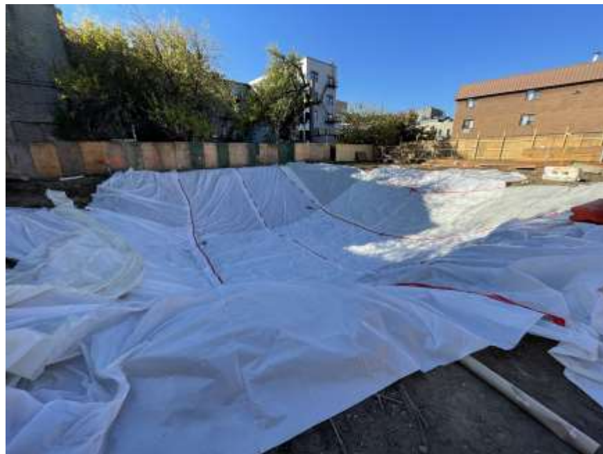
Photo 2: General view of the site at the end of the work day (facing northwest).
