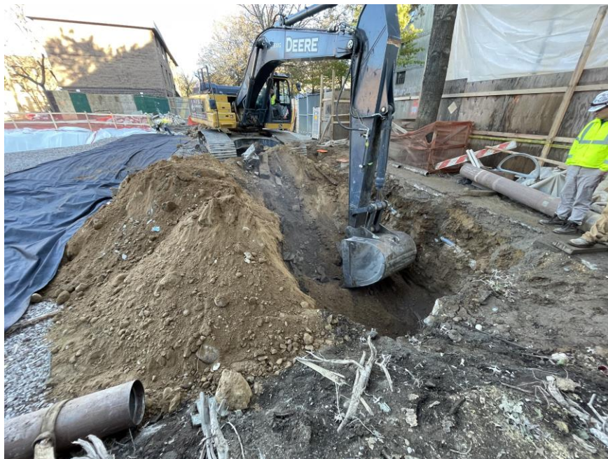
Photo 2: Rise excavating non-hazardous fill in the southwestern part of the site to remove subsurface obstructions (facing east).
