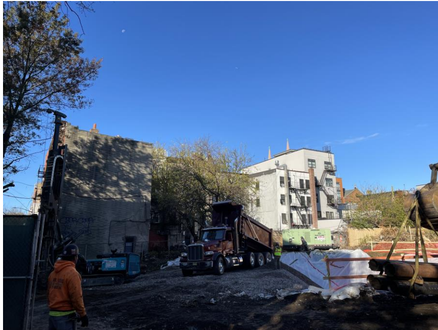
Photo 1: View of ¾-inch RCA imported for construction of the temporary equipment ramp in the central part of the site (facing northwest).
