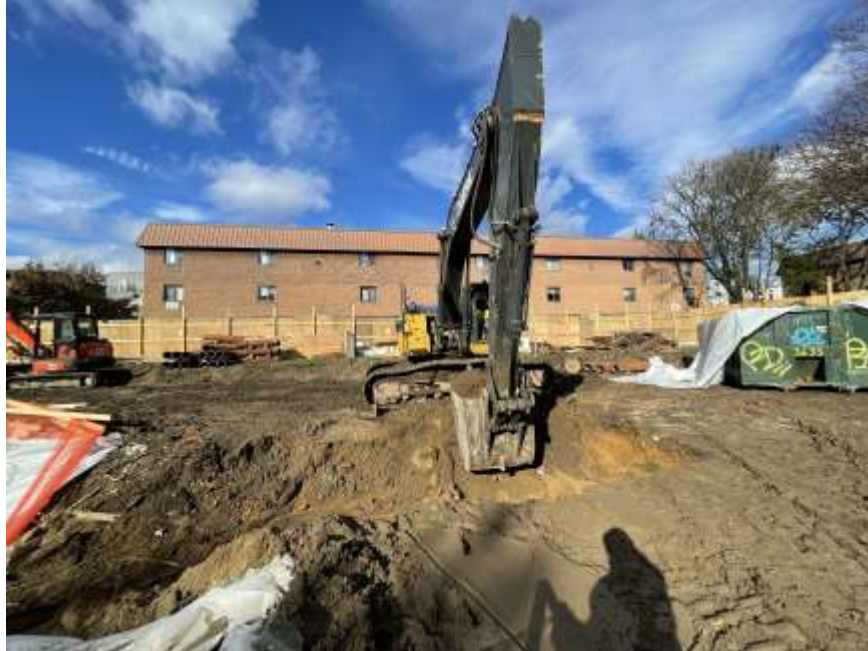
Photo 1: View of Rise excavating hazardous lead contaminated fill in the northeastern part of the site (facing north).
