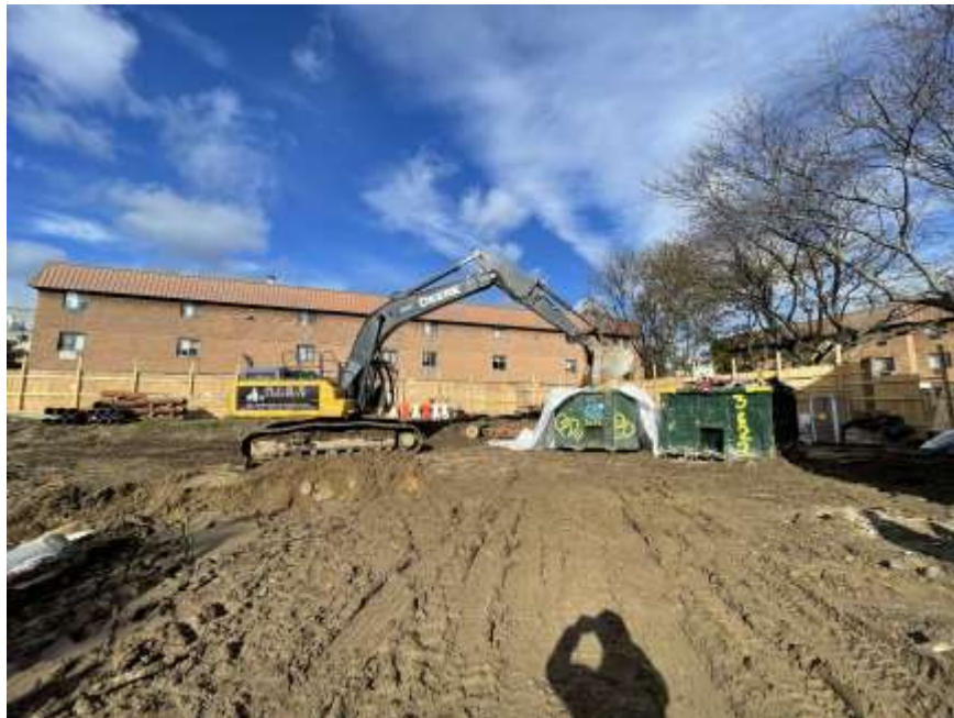
Photo 2: View of Rise containerizing hazardous lead contaminated fill in a polyethylene lined roll-off container in the northeastern part of the site (facing northeast).
