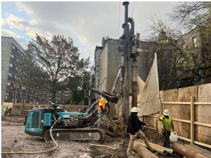
Photo 2: View of Anel drilling soldier piles along the western site boundary (facing northwest).
