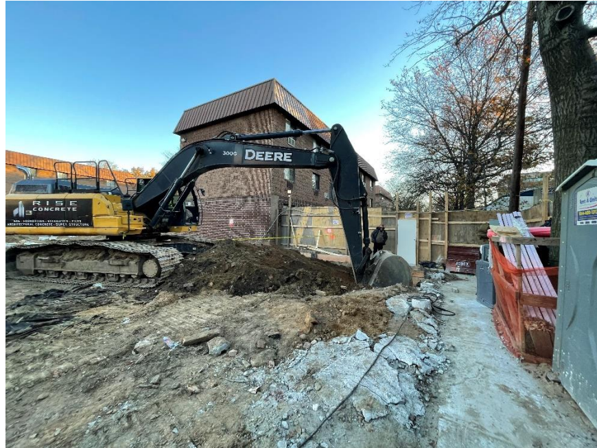
Photo 1: View of Rise excavating non-hazardous fill in the southeastern part of the site (facing northeast).
