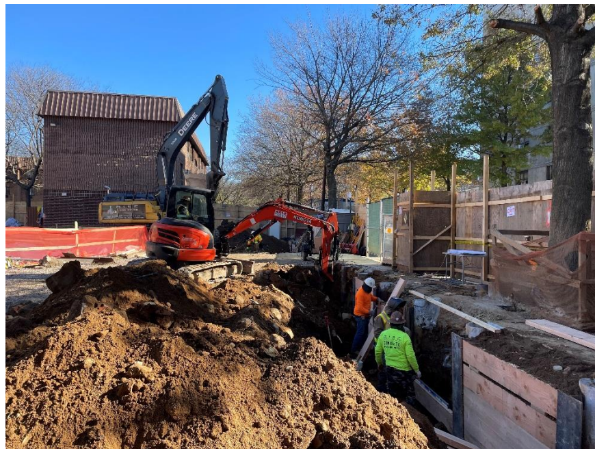
Photo 2: View of Rise installing lagging along the southern site boundary (facing east).
