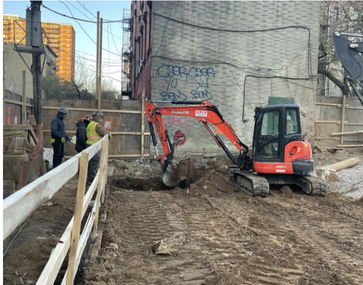
Photo 1: View of Rise excavating non-hazardous fill in the southwestern part of the site for SOE lagging installation (facing west).
