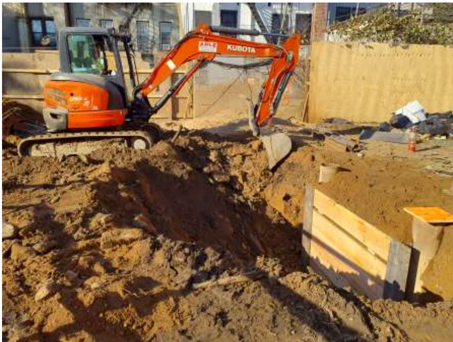
Photo 2: View of Rise excavating non-hazardous fill in the northwestern part of the site for SOE installation (facing west).
