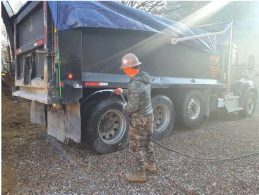
Photo 1: View of permitted tri-axle truck transporting non-hazardous fill for off-site disposal. Trucks were securely covered and tires washed prior to leaving the site (facing southeast).
