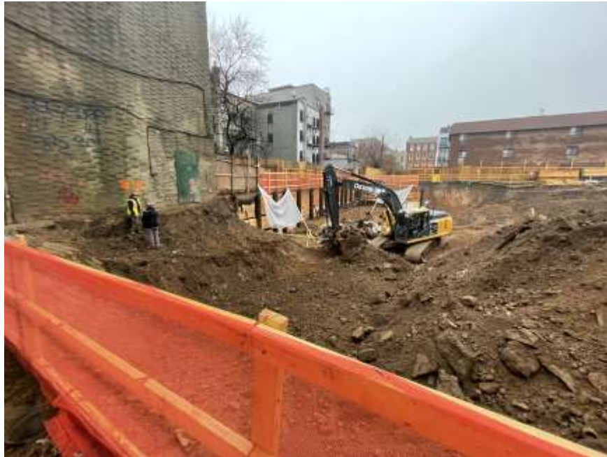
Photo 1: View of Rise excavating non-hazardous fill in the southwestern part of the site (facing northwest).
