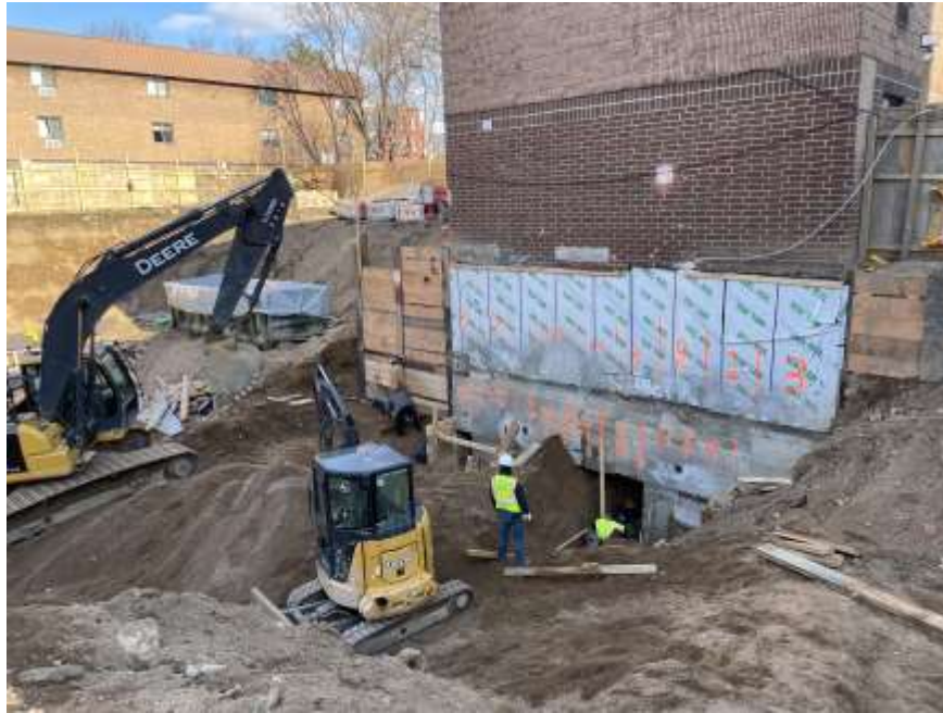
Photo 1: View of Rise excavating native soil for SOE underpinning installation (facing northeast).
