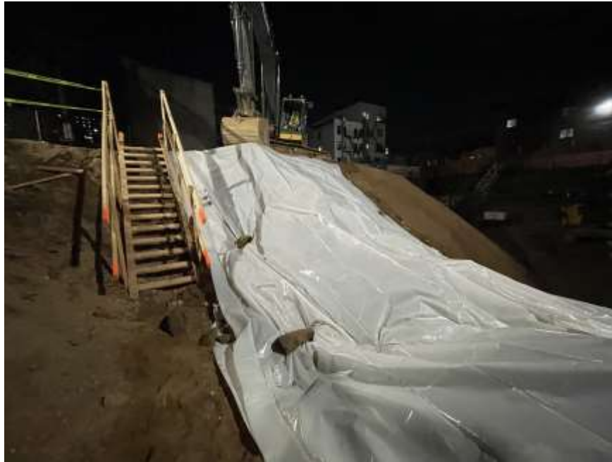
Photo 3: View of stockpiled hazardous lead contaminated soil on top of and covered with polyethylene sheeting in the southeastern part of the site (facing west).
