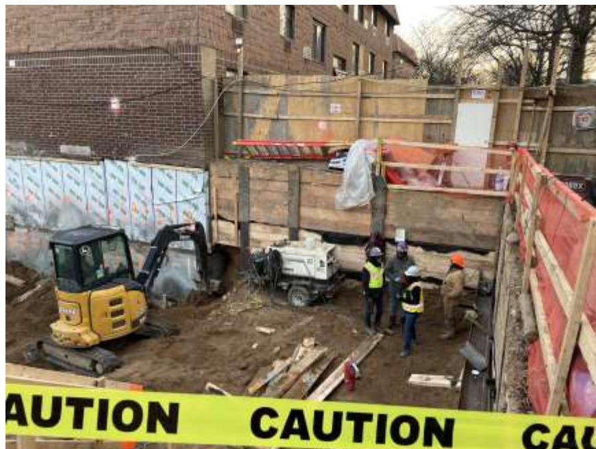
Photo 2: View of Rise excavating native soil for SOE underpinning installation in the southeastern part of the site (facing east).
