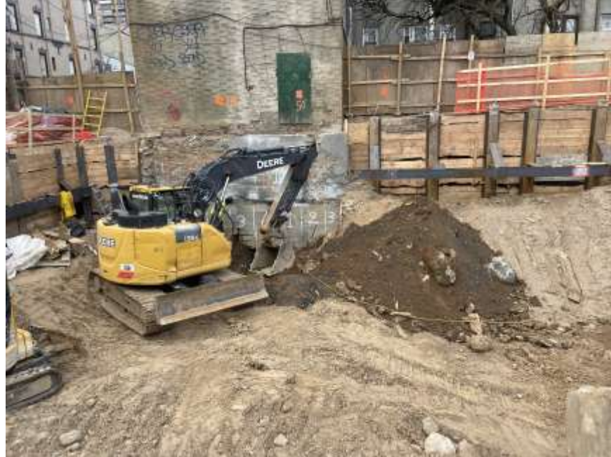
Photo 1: View of Rise excavating non-hazardous fill for SOE underpinning installation in the southwestern part of the site (facing west).
