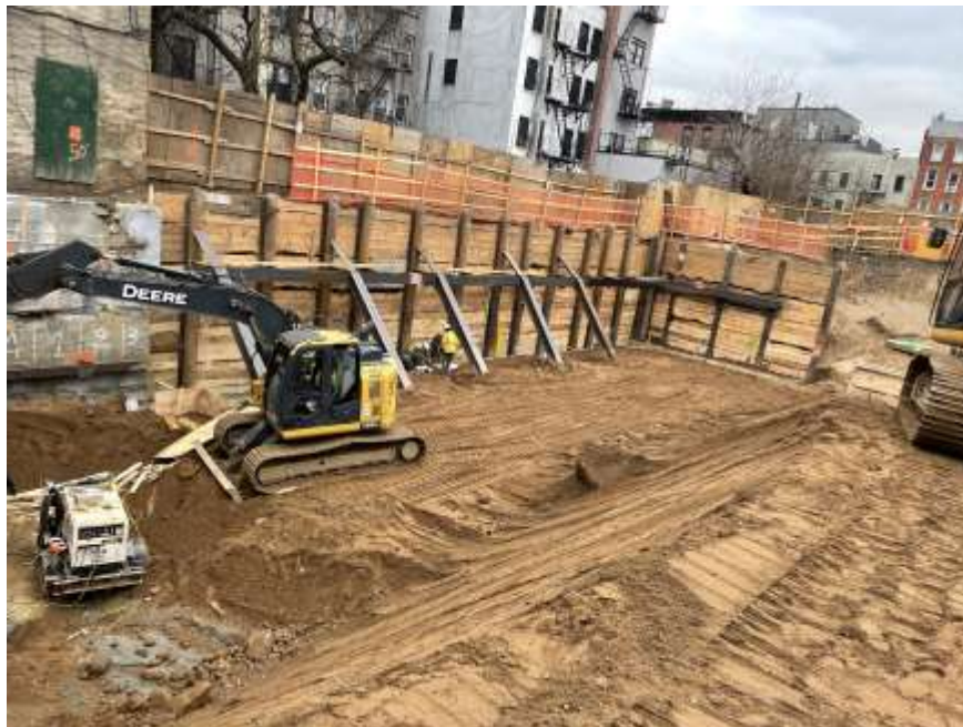
Photo 2: View of graded area in the western part of the site (facing northwest).
