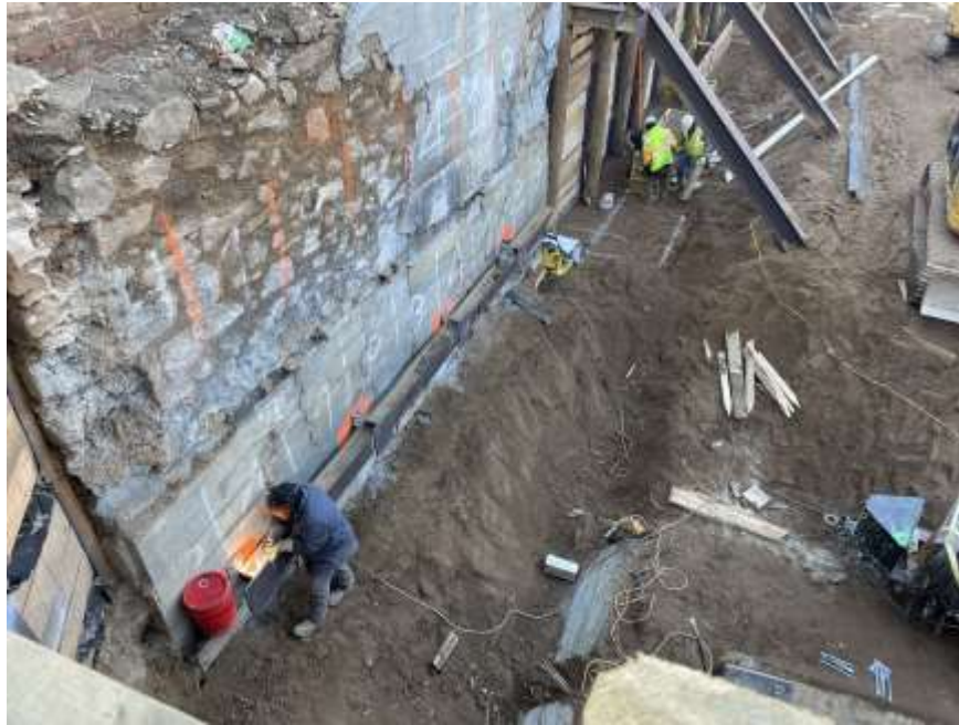
Photo 1: View of Rise installing SOE underpinning in the southwestern part of the site (facing northwest).
