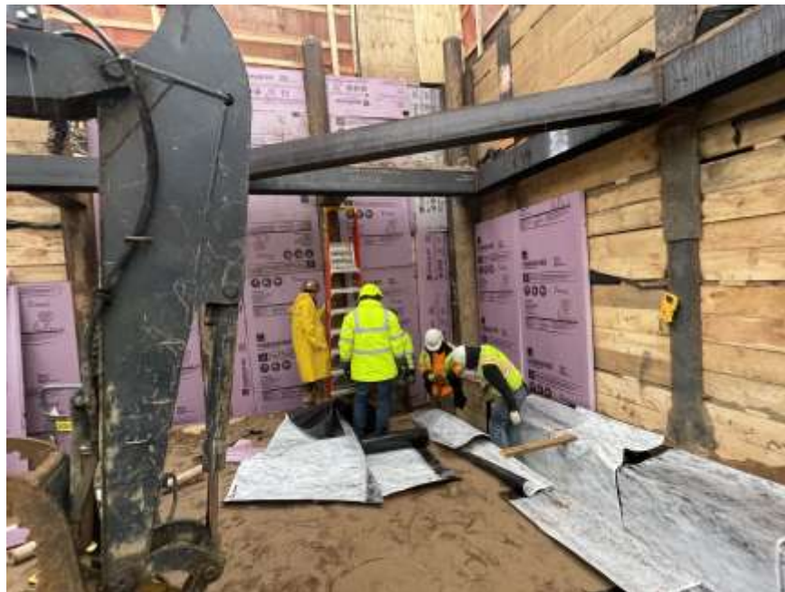
Photo 2: View of Rise installing Precon waterproofing in the northwest part of the site (facing norhtwest).
