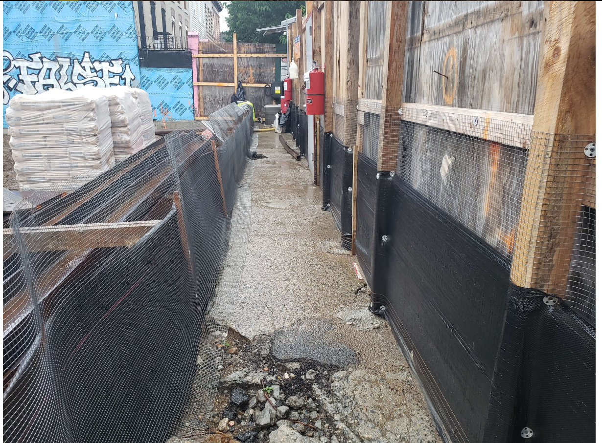
Photo 2 – View of sidewalk between Bayard property boundary and construction fence. No sediment runoff
