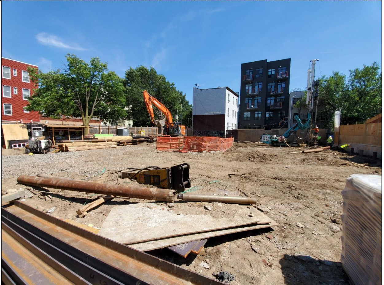
Photo 4 – Site at end of the day, view is facing south from site entrance on Bayard St.
