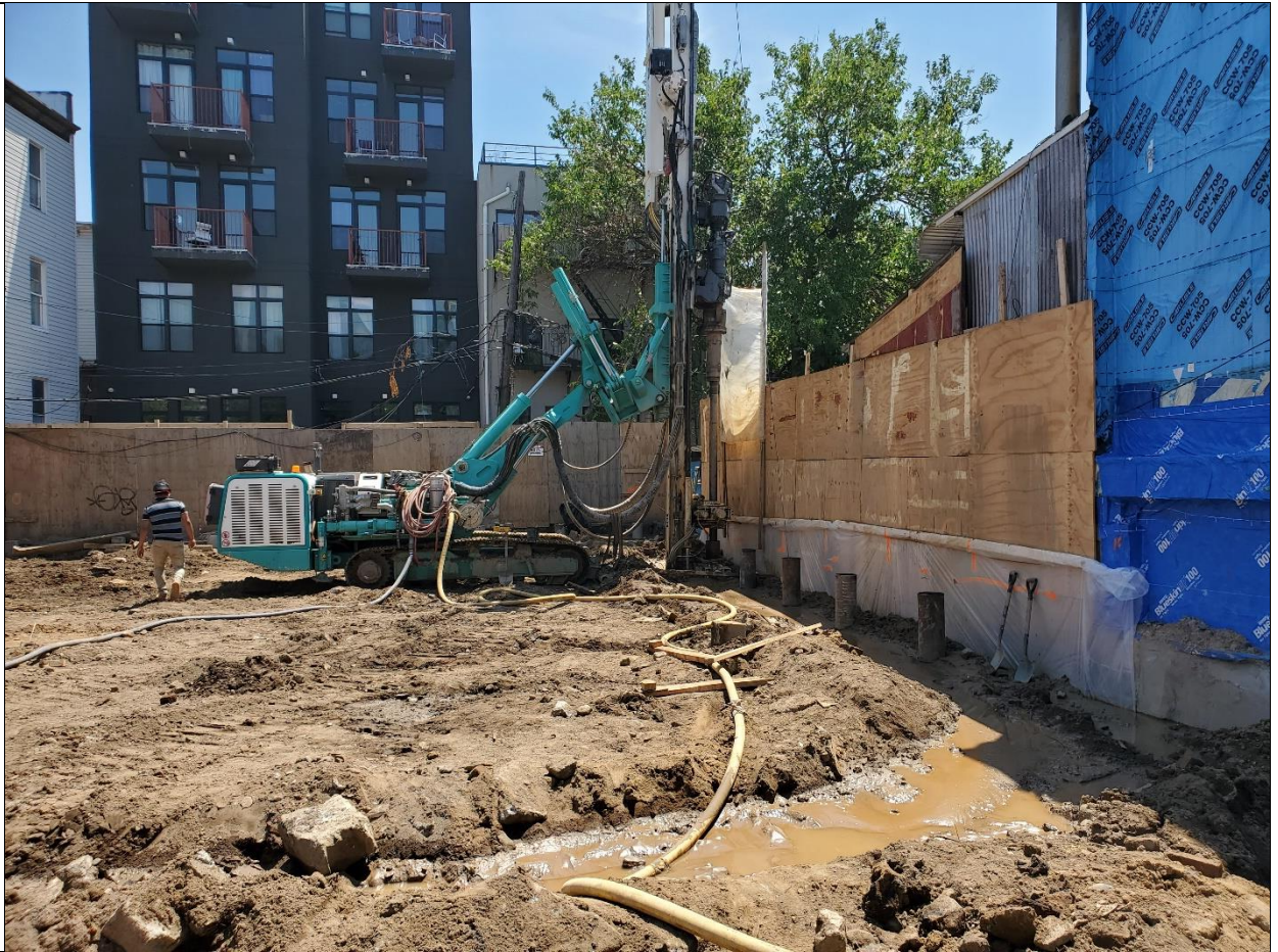
Photo 3 – Piles being driven using water at west side of Grid A3. Five piles driven, view is facing west in Grid A3 towards neighboring property.
