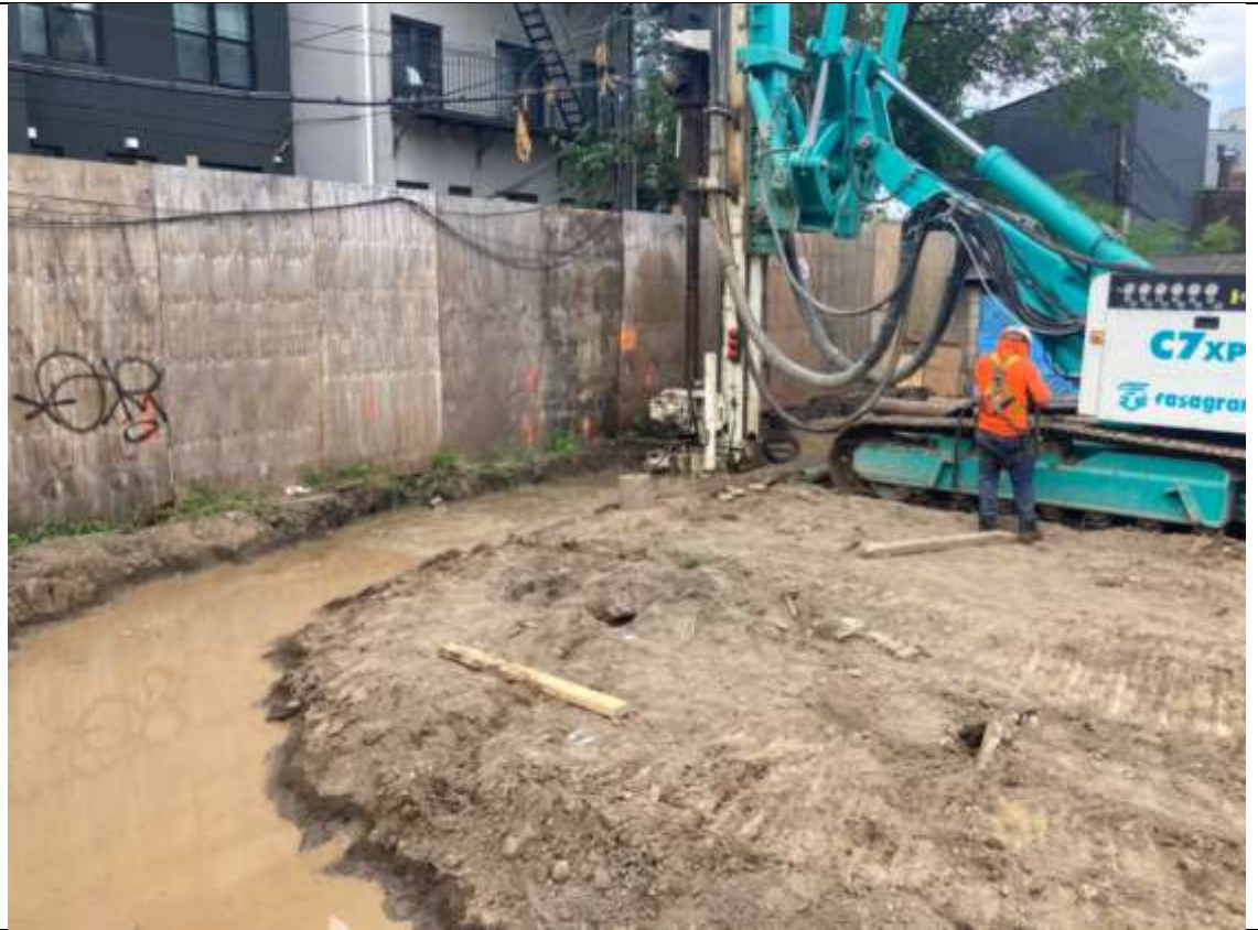
Photo 3 – Pile drilling in Grid A3 adjacent to lot 27. A trench was dug to allow excess water to drain in to the elevator pit.
