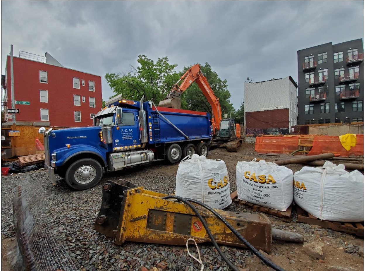
Photo 2 – Truck being loaded with soil from (0-5') to be sent to Former New Jersey Zinc- West Plant, Palmerston PA. View is facing southeast from site entrance on Bayard St.
