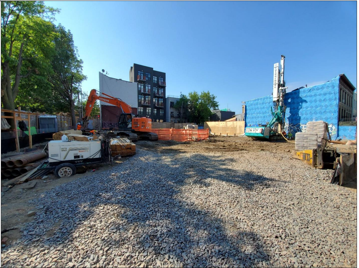
Photo 1 – Site at beginning of the day, view is facing south from site entrance on Bayard St.
