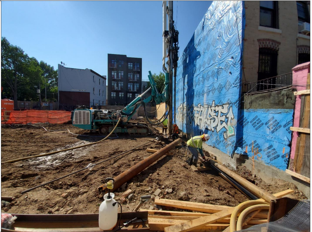
Photo 3 – Additional view of piles being driven with water at west side of site along neighboring property on Bayard St, view is facing south in Grid A1.
