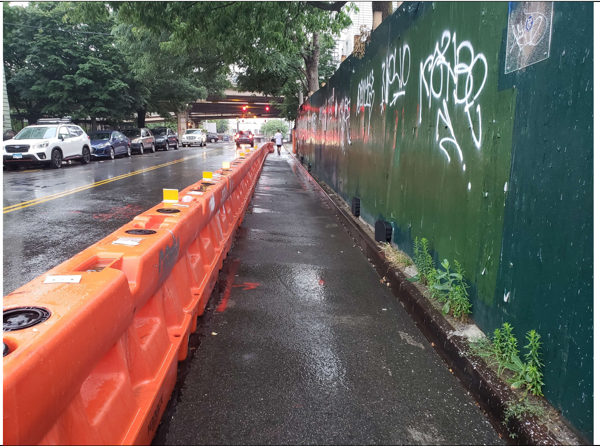
Photo 3 – View of Graham avenue along exterior of construction fence during rain. No sediment runoff
