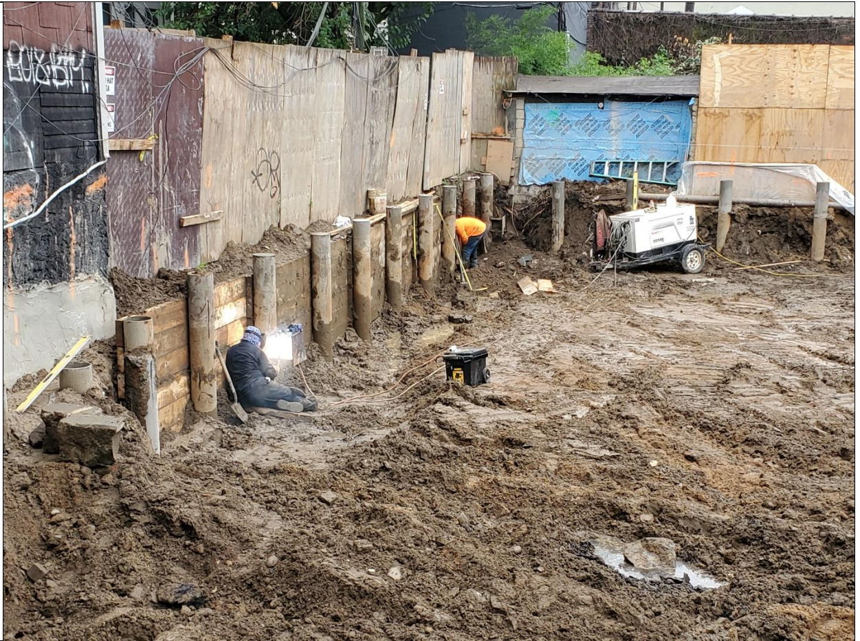
Photo 3 – Lagging installed to 5' bsg and welding for SOE at south side of grids A3 and B3. View is facing west from Graham Ave.
