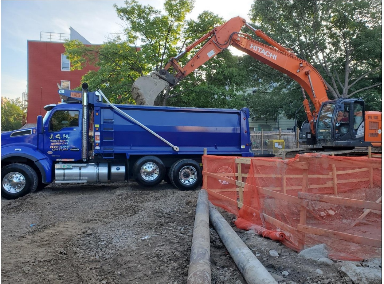
Photo 2 – Truck being loaded with soil from (0-5') to be sent to Former New Jersey Zinc- West Plant, Palmerston PA. View is facing east towards Graham Ave.
