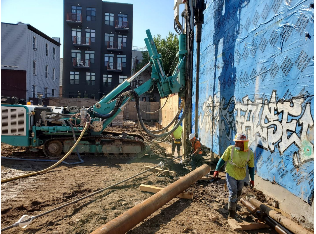
Photo 2 – Piles being driven with water at west side of site in Grid A1, view is facing south towards Lot 27.
