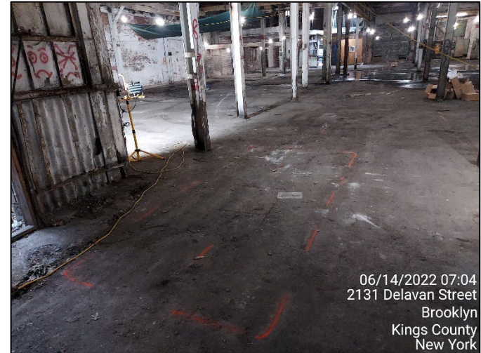
Photograph 2: A metallic anomaly (suspected UST) in the southern portion of the warehouse. (June 2022)
