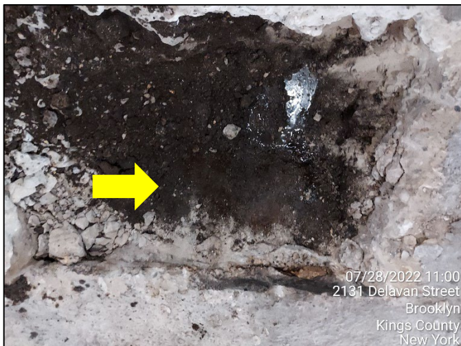
Photograph 21: Confirmation of an UST at the magnetic anomaly that was identified in the southern portion of the warehouse. (July 2022)
