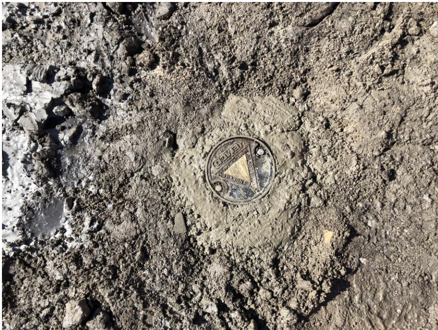
Photo 12, 5/13/2020: View of the flush-mount cover installed over monitoring well MW16.
