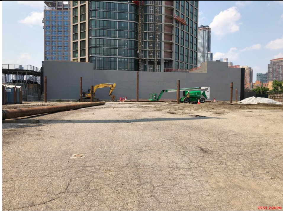
Photo 1: View of index piles installed in the central part of the site (facing north).
