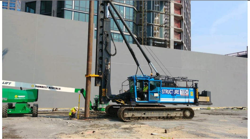
Photo 1: View of STNY installing an index pile at the northeastern corner of the site (facing north).
