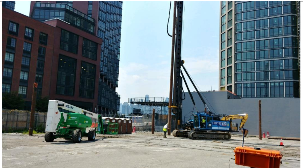
Photo 2: View of a completed index pile in the western part of the site (facing northwest).
