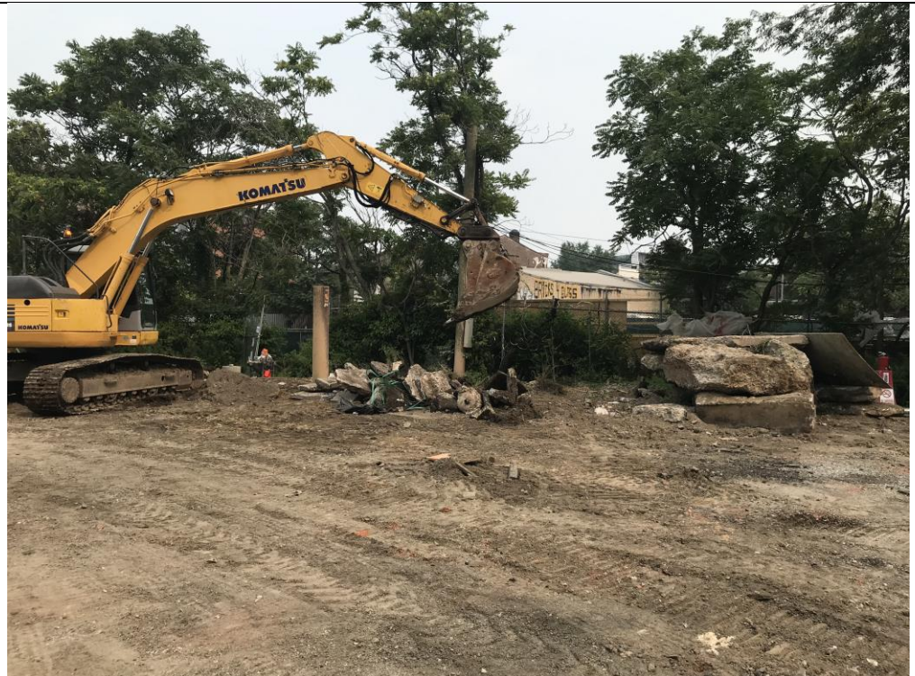
Photo 4: View of STNY relocating soil and concrete stockpiles within COMP A (facing south)
