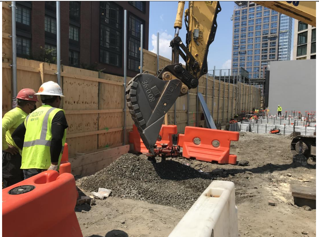
Photo 4: View of STNY backfilling utility trenches in waste characterization grid COMP G (facing north).
