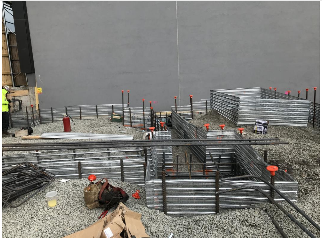
Photo 4: View of backfilled area and pile cap formwork in waste characterization grid COMP E (0-5) (facing north).
