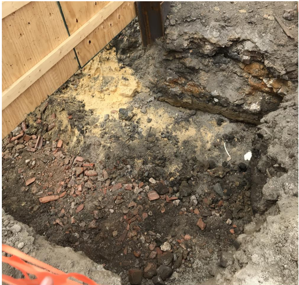
Photo 4: View of water utility pipe excavation in waste characterization grid COMP G (0-5) (facing west).
