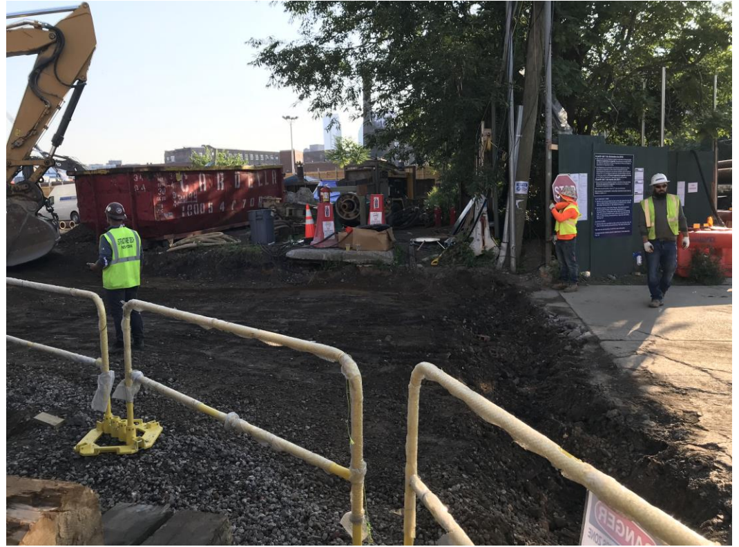
Photo 2: View of truck pad excavation in waste characterization grids COMP H (0-5) and COMP J South (0-2) (facing east)
