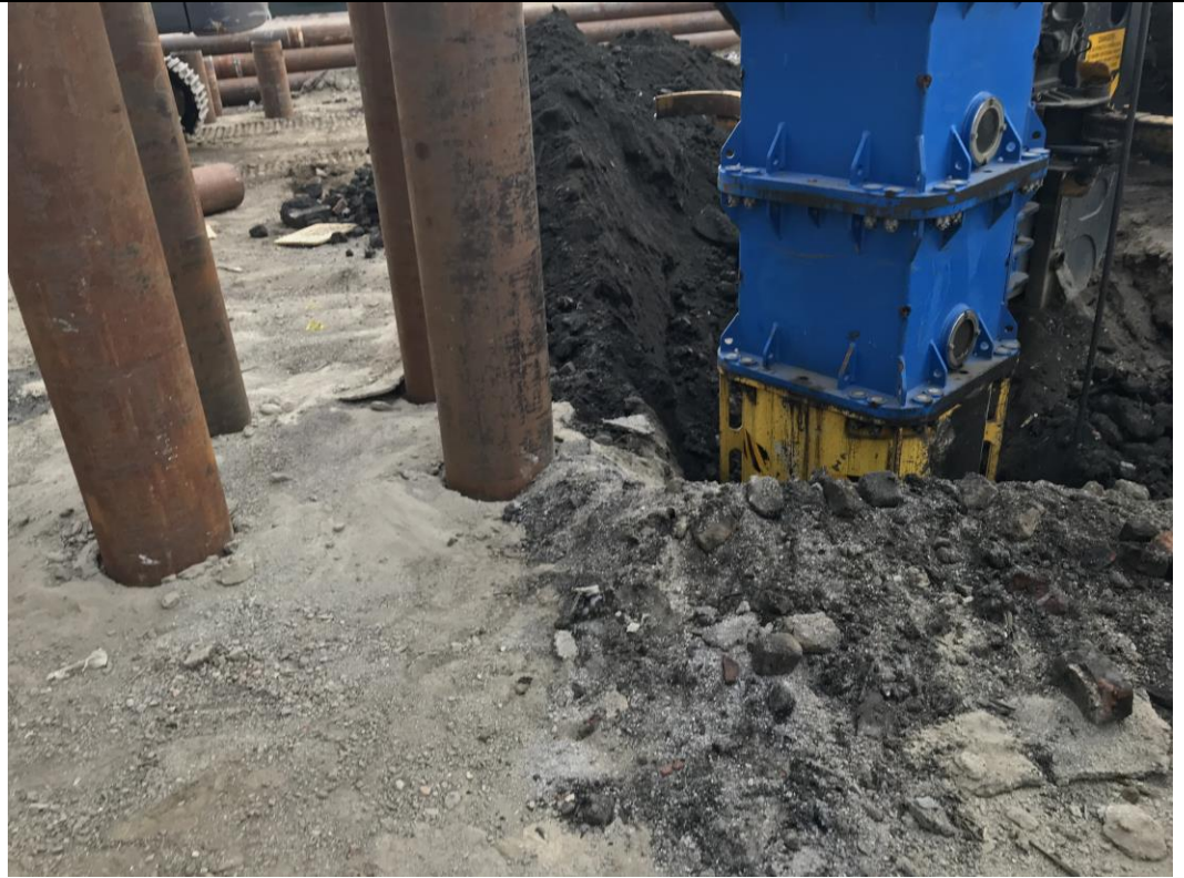
Photo 3: View of pile excavation in waste characterization grid COMP C (0-5) (facing east).
