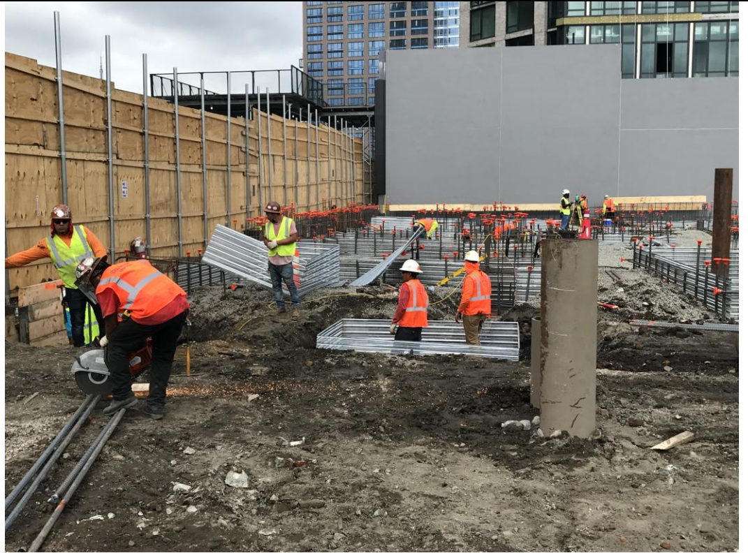
Photo 3: View of STNY installing formwork in waste characterization grid COMP F (facing north).
