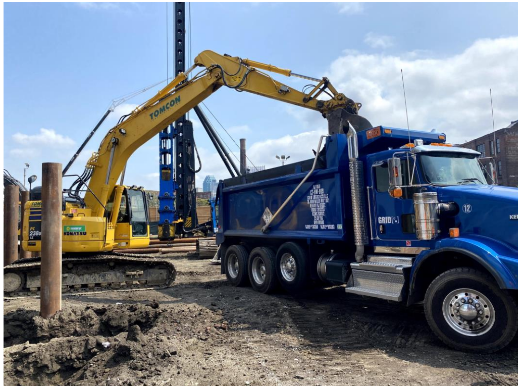
Photo 4: View of STNY excavating hazardous lead hotspot LB22 and live loading onto trucks for off-site disposal (facing east).
