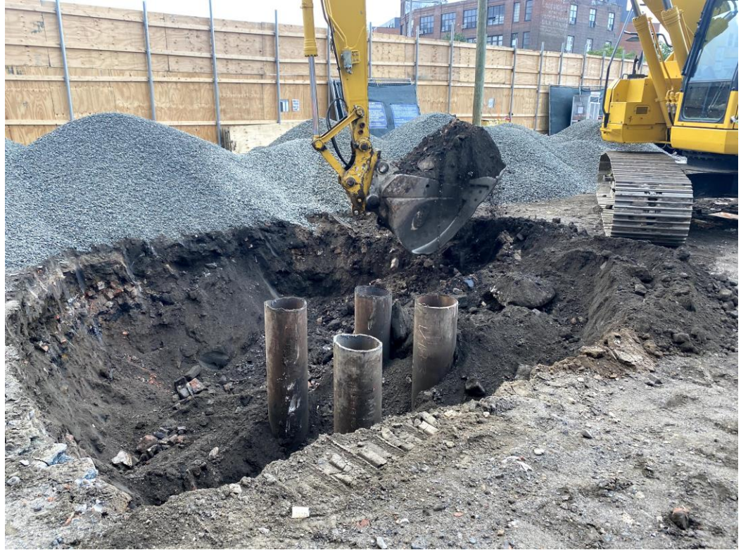
Photo 3: View of STNY excavating hazardous lead hotspot LB17 for export and off-site disposal (facing east).
