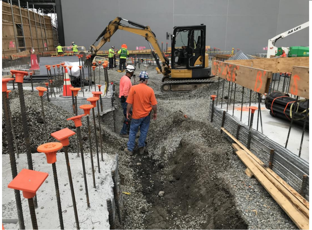
Photo 3: View of STNY excavating for plumbing in waste characterization grid COMP F (facing north).
