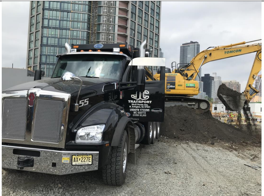
Photo 4: View of STNY loading a truck with soil for off-site disposal to CEPA (facing north).
