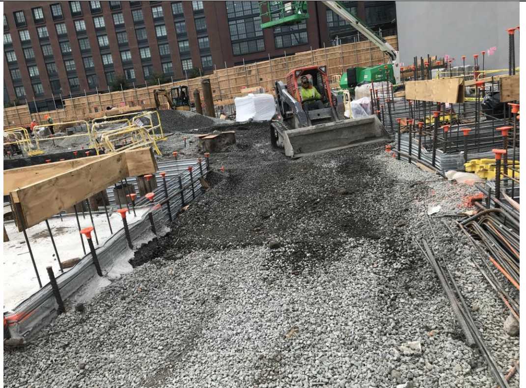
Photo 1: View of STNY backfilling with 0.75-inch virgin stone in waste characterization grid COMP C (facing east).
