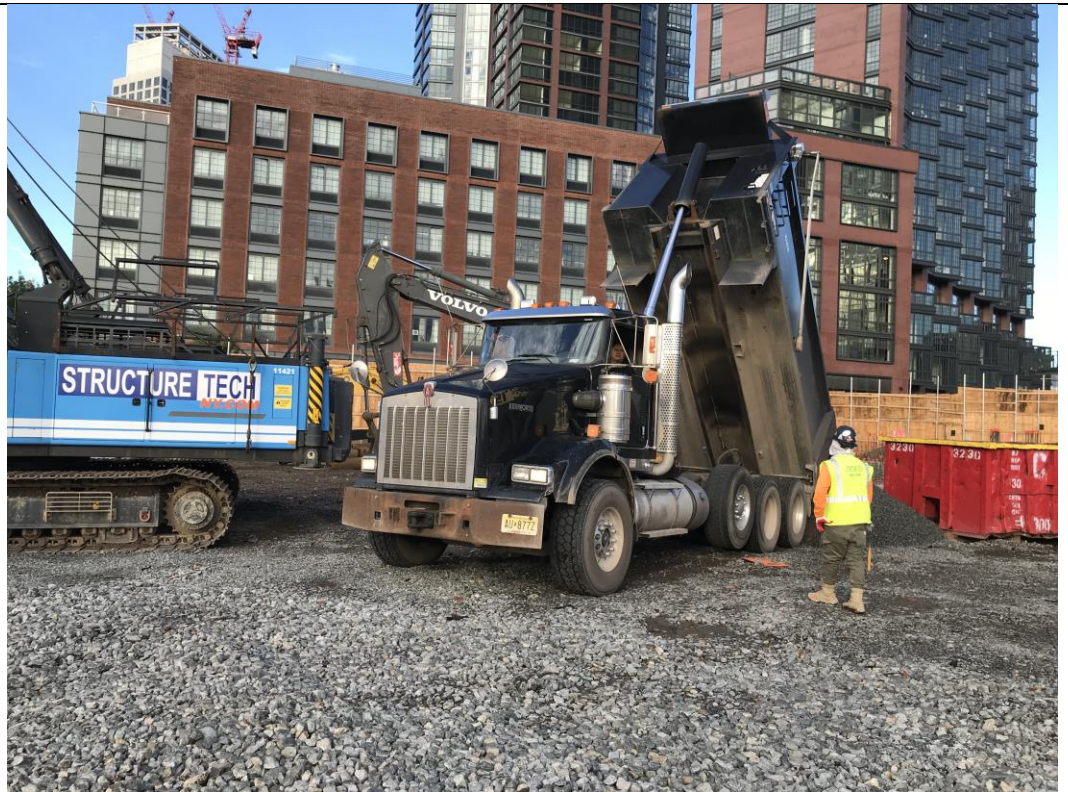
Photo 4: View of truck dumping imported 0.75-inch virgin stone from Tilcon - Mt. Hope Quarry (facing west).
