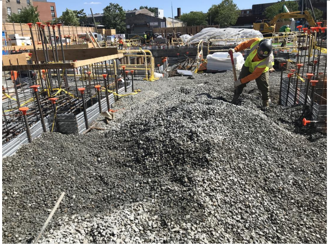
Photo 3: View of STNY backfilling with imported 0.75-inch virgin stone in waste characterization grid COMP C (facing south).
