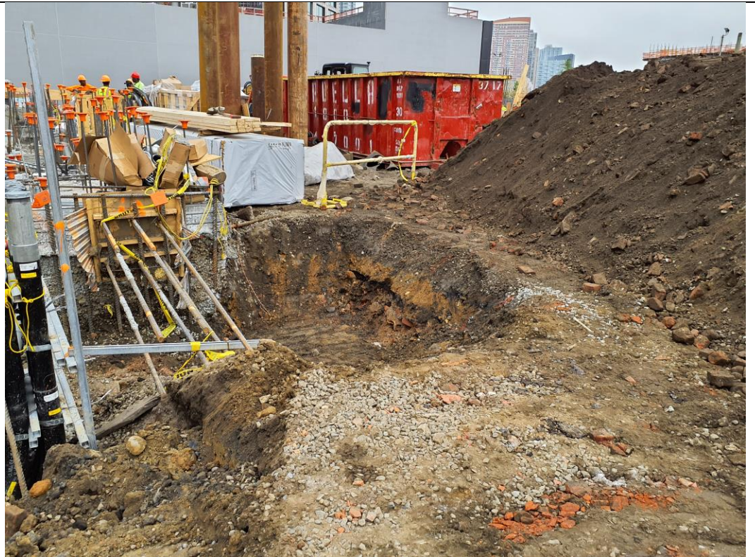
Photo 2: View of electric utility piping excavation in waste characterization grid COMP J South (facing northeast).
