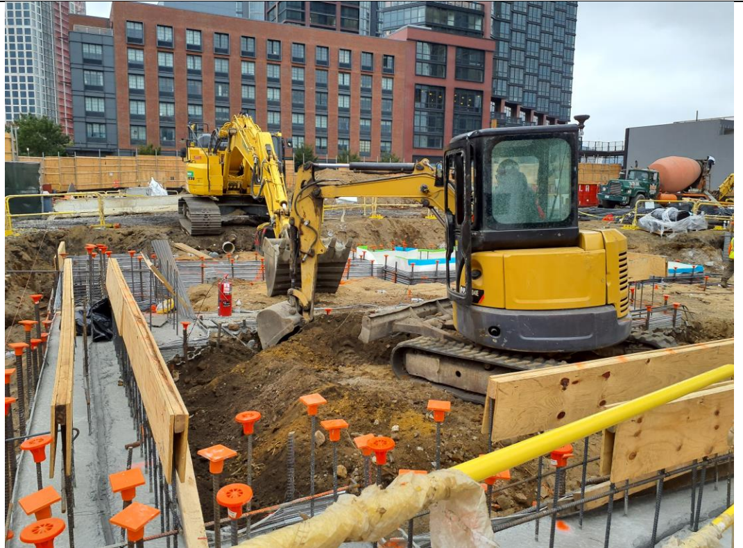
Photo 1: View of STNY excavating previously placed backfill in waste characterization grid COMP A (facing west).
