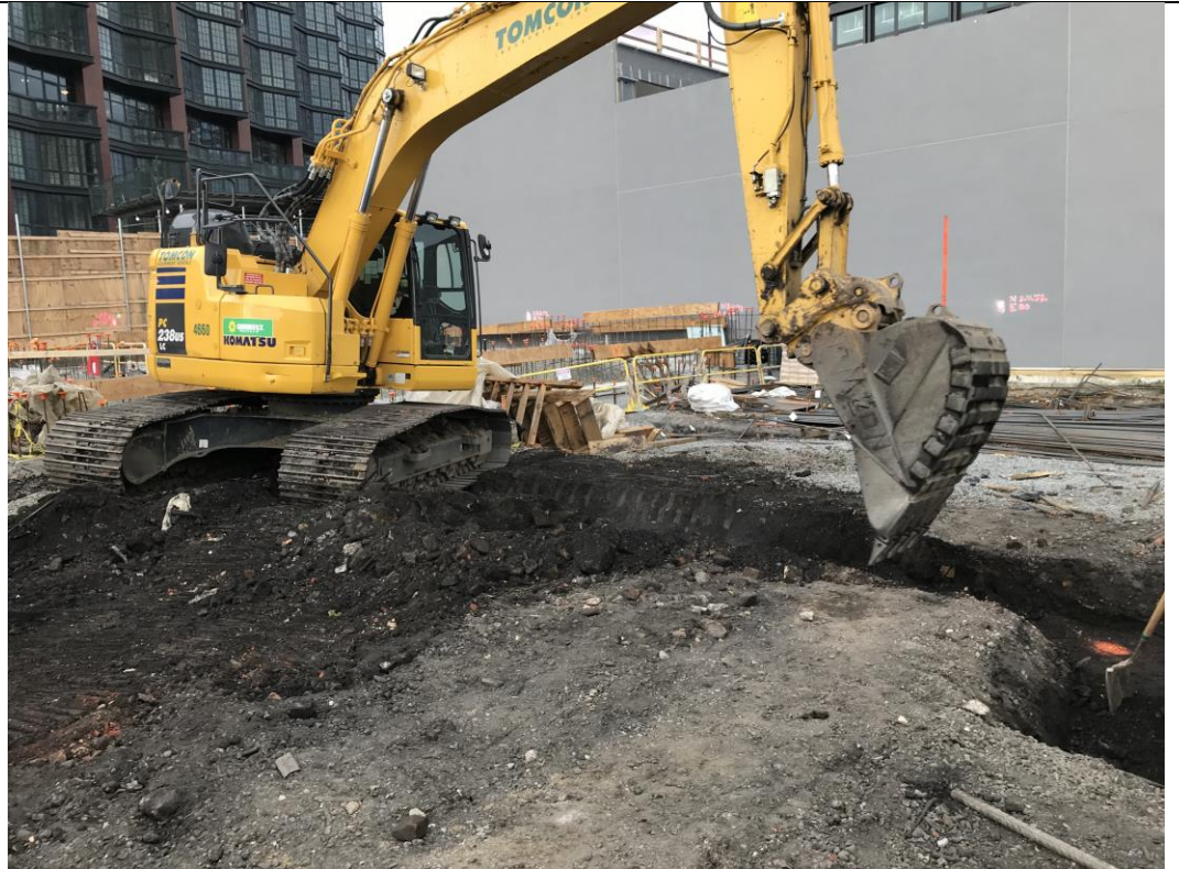
Photo 1: View of STNY excavating for pile cap and grade beam formwork in waste characterization grid COMP D (facing northwest).
