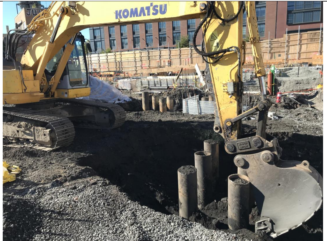
Photo 1: View of STNY excavating for pile cap and grade beam formwork installation in waste characterization grid COMP D (facing west).
