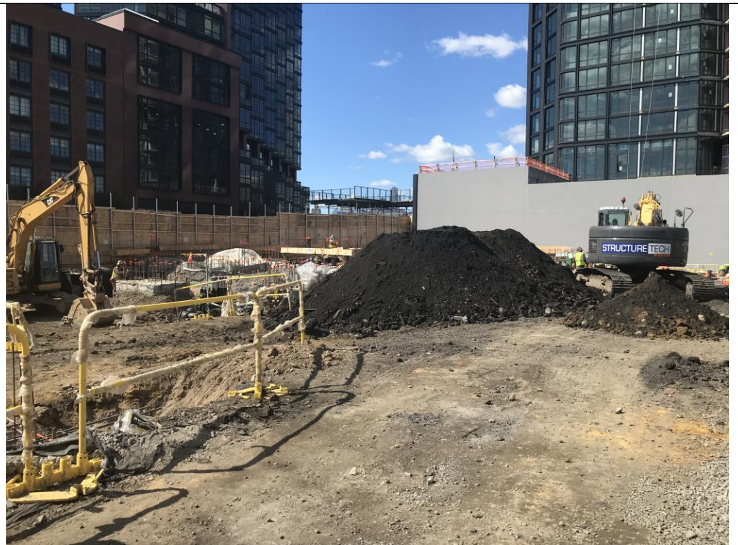
Photo 2: View of STNY relocating Soil Stockpile 1 in waste characterization grid COMP J South (facing north).
