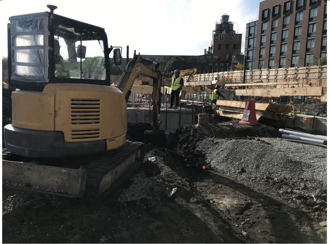
Photo 3: View of plumbing excavation in waste characterization COMP J North (facing west).
