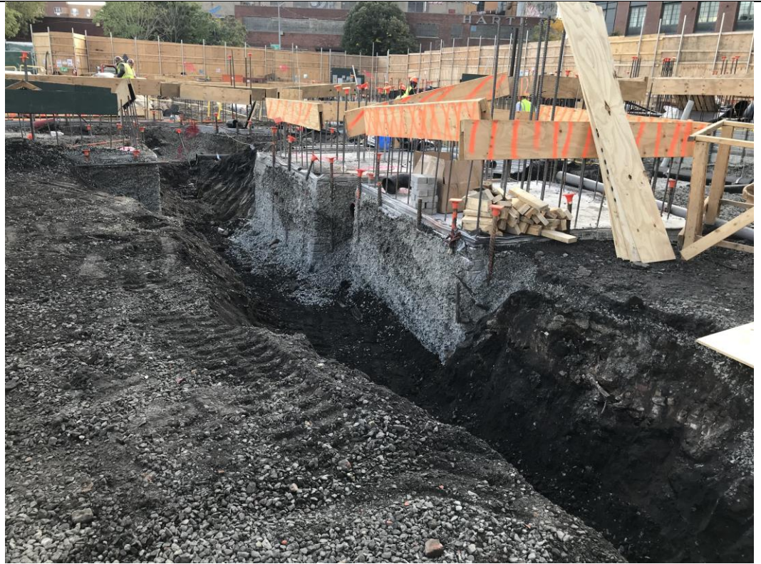
Photo 4: View of plumbing excavation in waste characterization grid COMP D (facing southwest).
