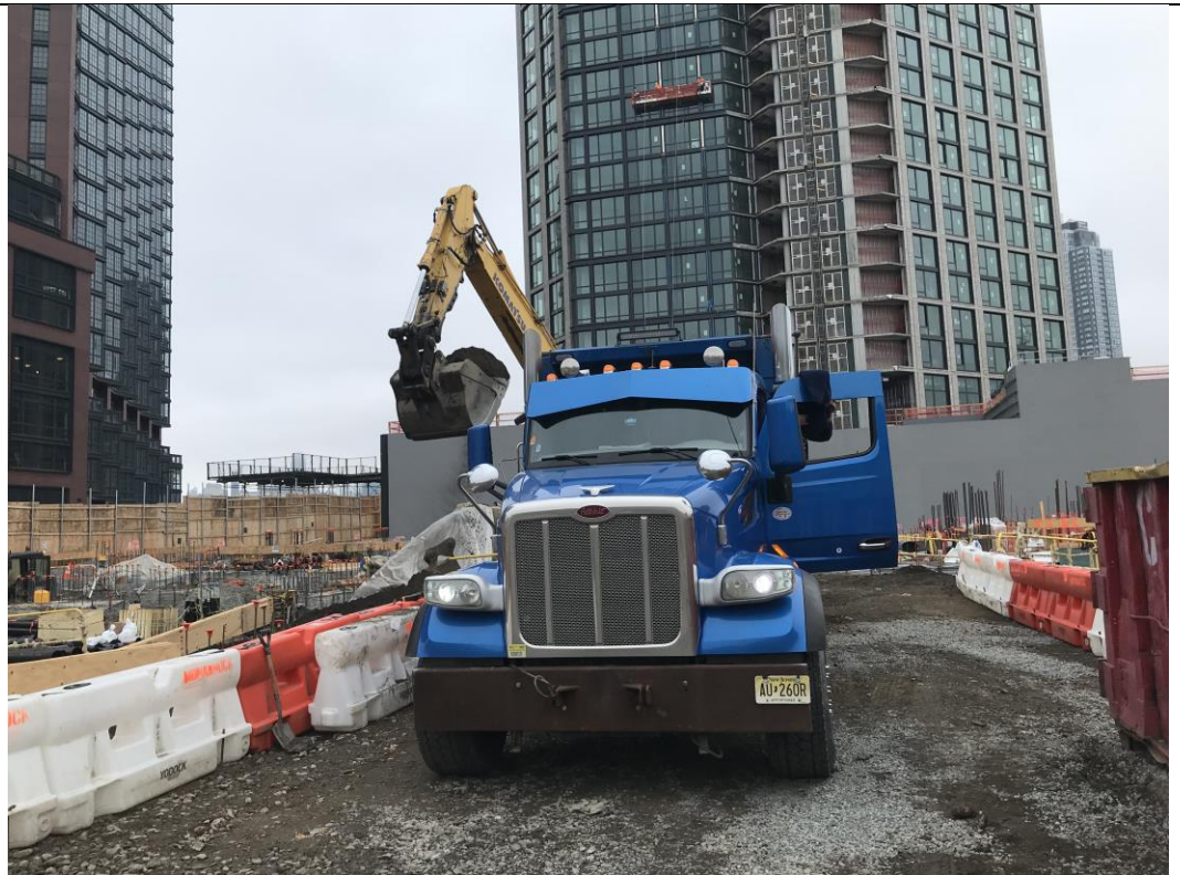
Photo 4: View of STNY loading soil into trucks for off-site disposal to the CEPA facility (facing north).
