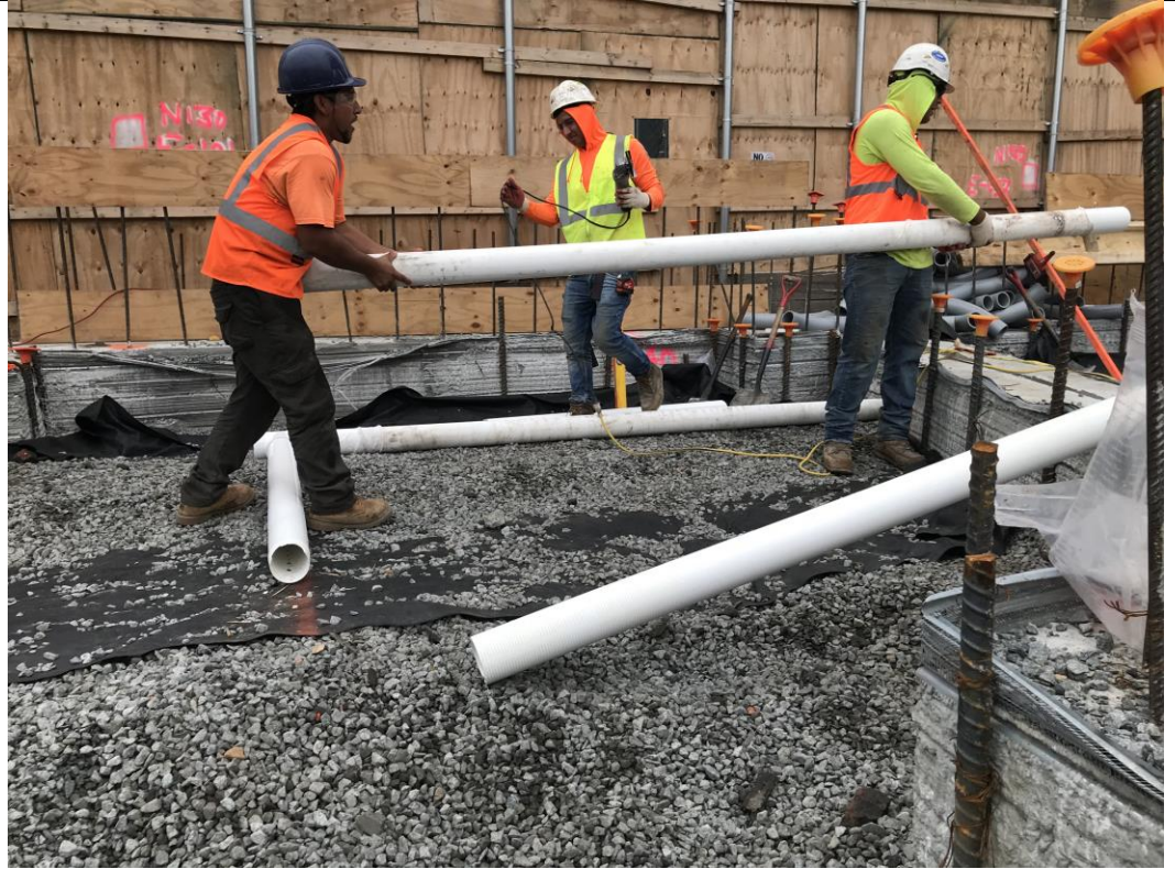
Photo 3: View of STNY installing PVC piping for the SMD system in waste characterization grid COMP F (facing west).
