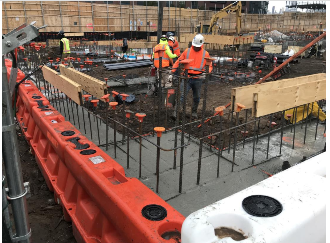
Photo 2: View of STNY pouring concrete for grade beams in waste characterization grid COMP H (facing northwest).
