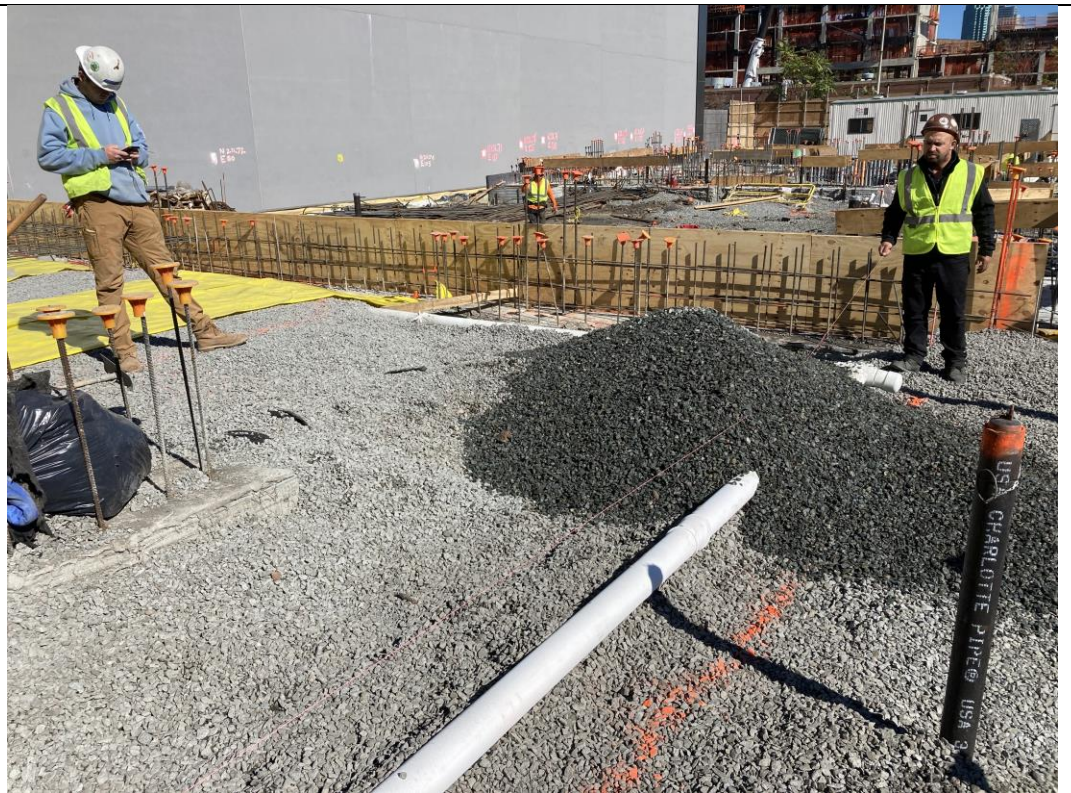
Photo 2: View of STNY installing SMD piping and aggregate layer in waste characterization COMP E (facing northeast).
