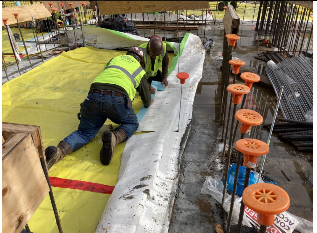
Photo 1: View of STNY installing vapor barrier in waste characterization grid COMP C (facing north).
