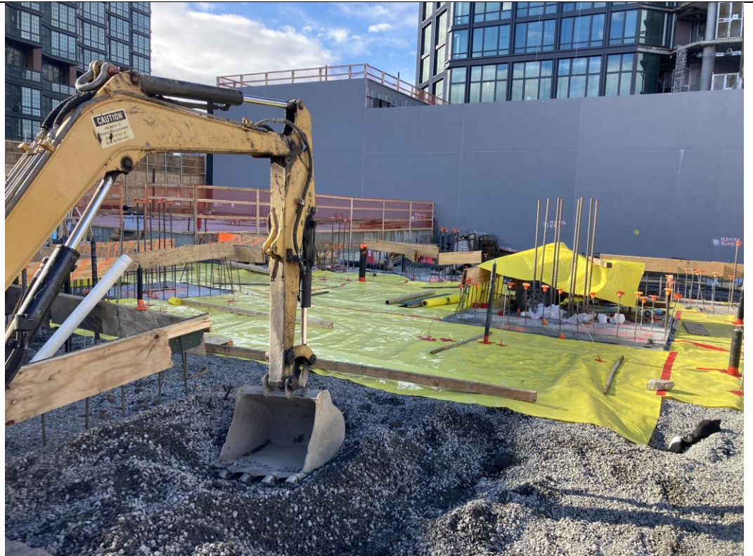
Photo 2: View of installed vapor barrier in waste characterization grid COMP D (facing northwest).
