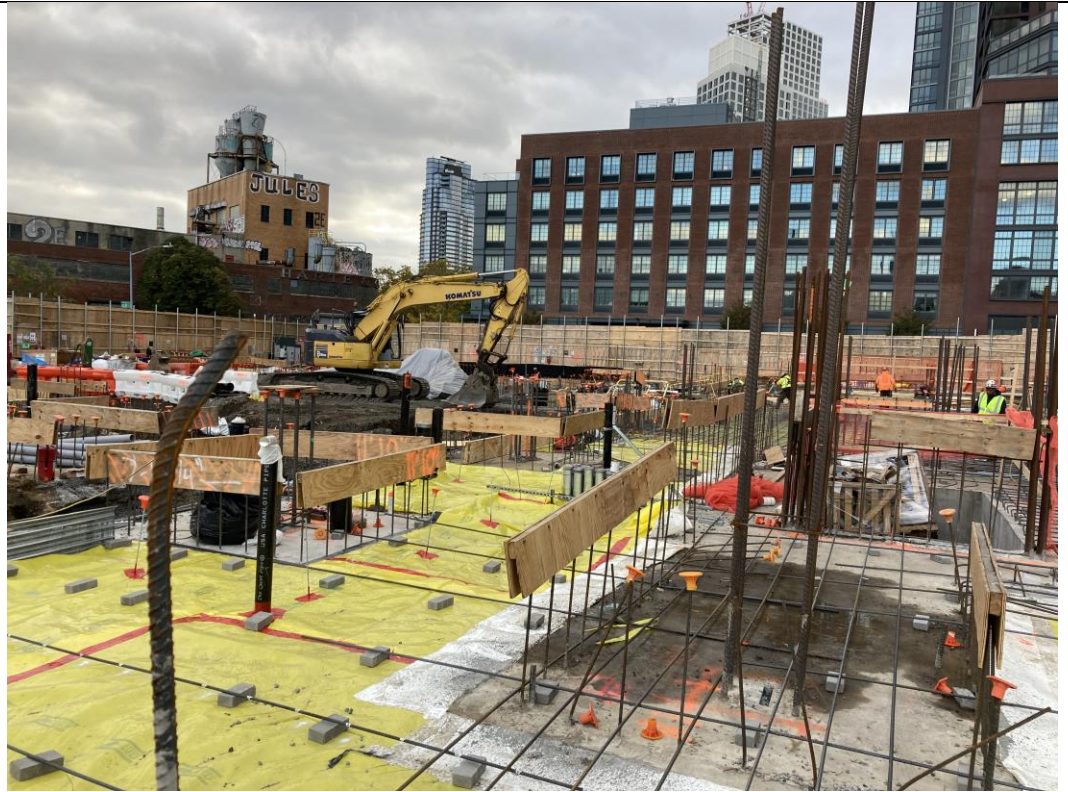
Photo 4: General view of the site and installed vapor barrier in waste characterization grids COMP B and COMP D at the end of the workday (facing southwest).
