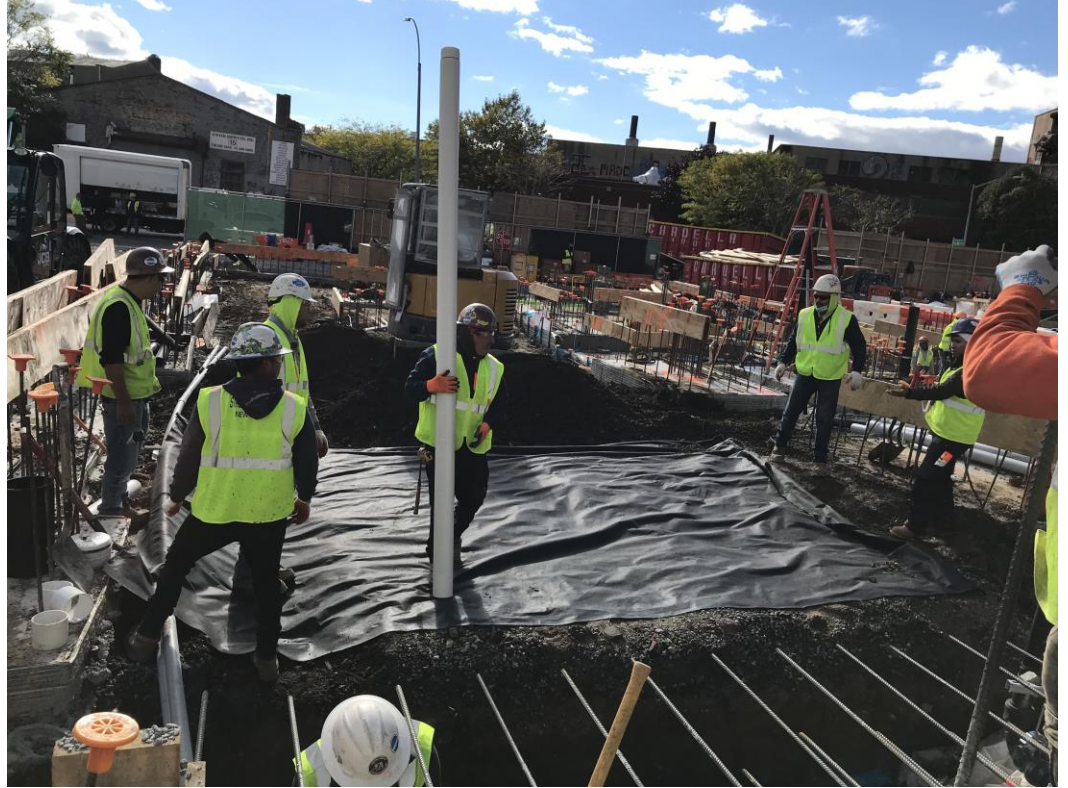
Photo 3: View of STNY placing geotextile fabric (Mirafi 140N) for the SMD system in waste characterization grid COMP B (facing south)
