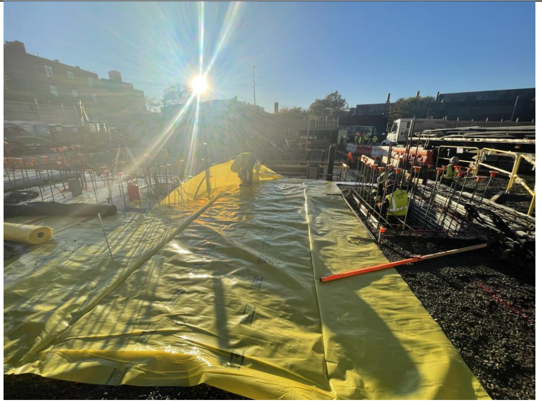
Photo 4: General view of vapor barrier installation in waste characterization grid COMP B (facing south).
