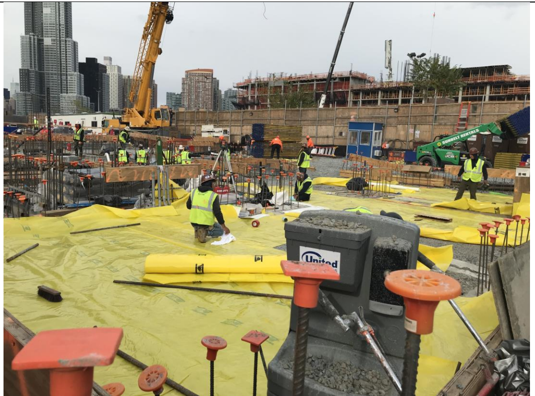
Photo 4: View of STNY placing vapor barrier in waste characterization grid COMP A (facing north)
