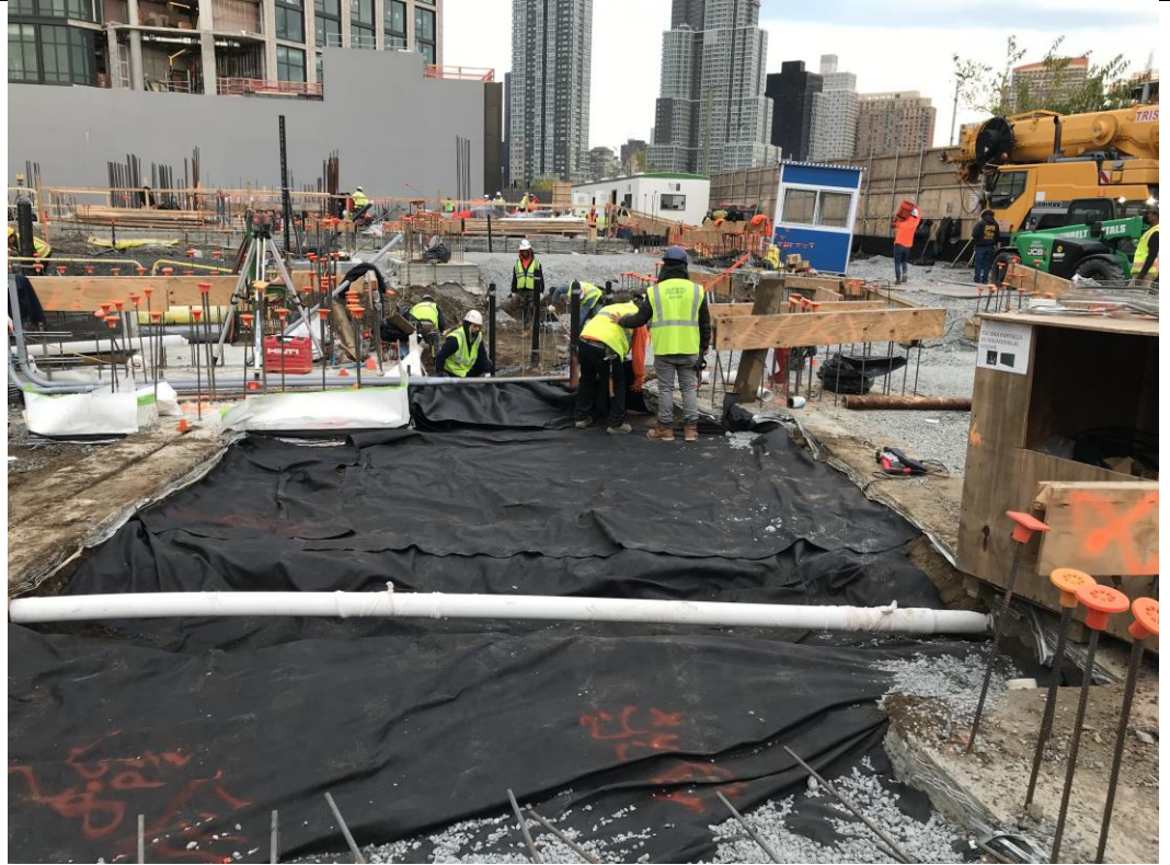
Photo 3: View of STNY placing geotextile fabric (Mirafi 140N) for the SMD system in waste characterization grid COMP A (facing north).
