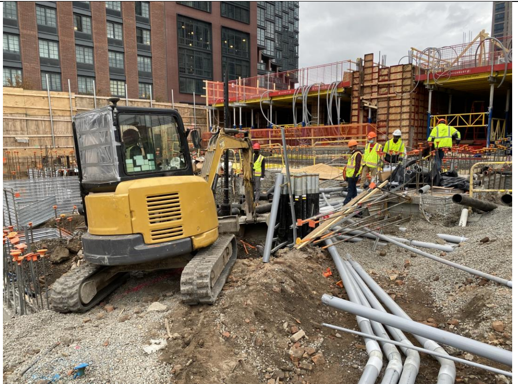
Photo 2: View of STNY excavating in waste characterization grid COMP J South to install electrical utilities (facing west).
