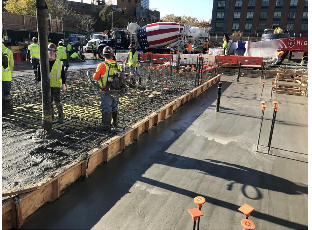
Photo 1: View of STNY pouring concrete foundation in waste characterization grid COMP A (facing west).
