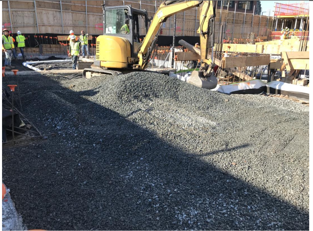
Photo 4: View of STNY backfilling with imported stone for the SMD system in waste characterization grid COMP H (facing northwest).
