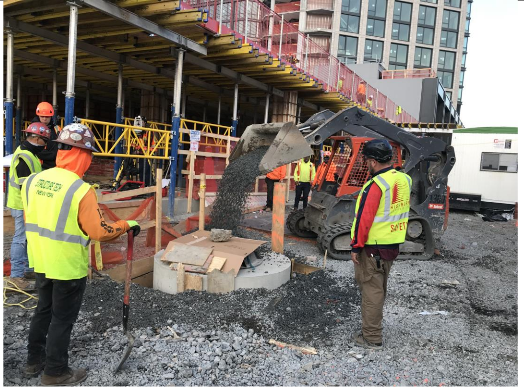
Photo 3: View of STNY backfilling with imported stone in waste characterization grid COMP K (facing north).
