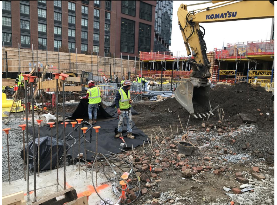
Photo 3: View of STNY regrading/flattening an area in waste characterization grid COMP H in preparation for installation of SMD system components (facing northwest).
