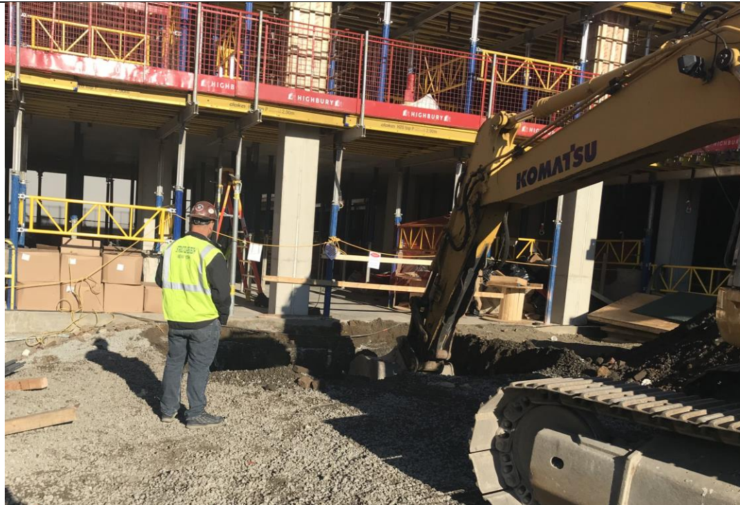
Photo 2: View of STNY excavating in waste characterization grid COMP J South (facing northeast)
