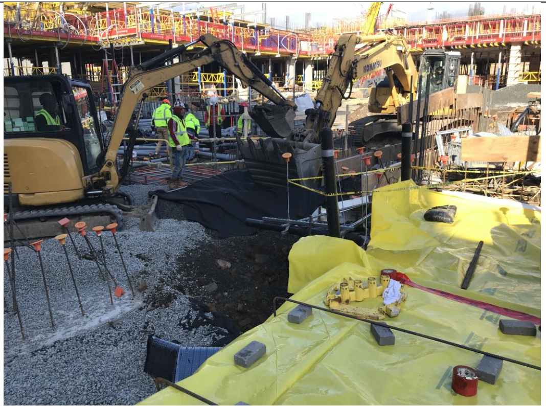
Photo 4: View of STNY excavating in waste characterization area COMP H for pile cap formwork installation (facing northeast).
