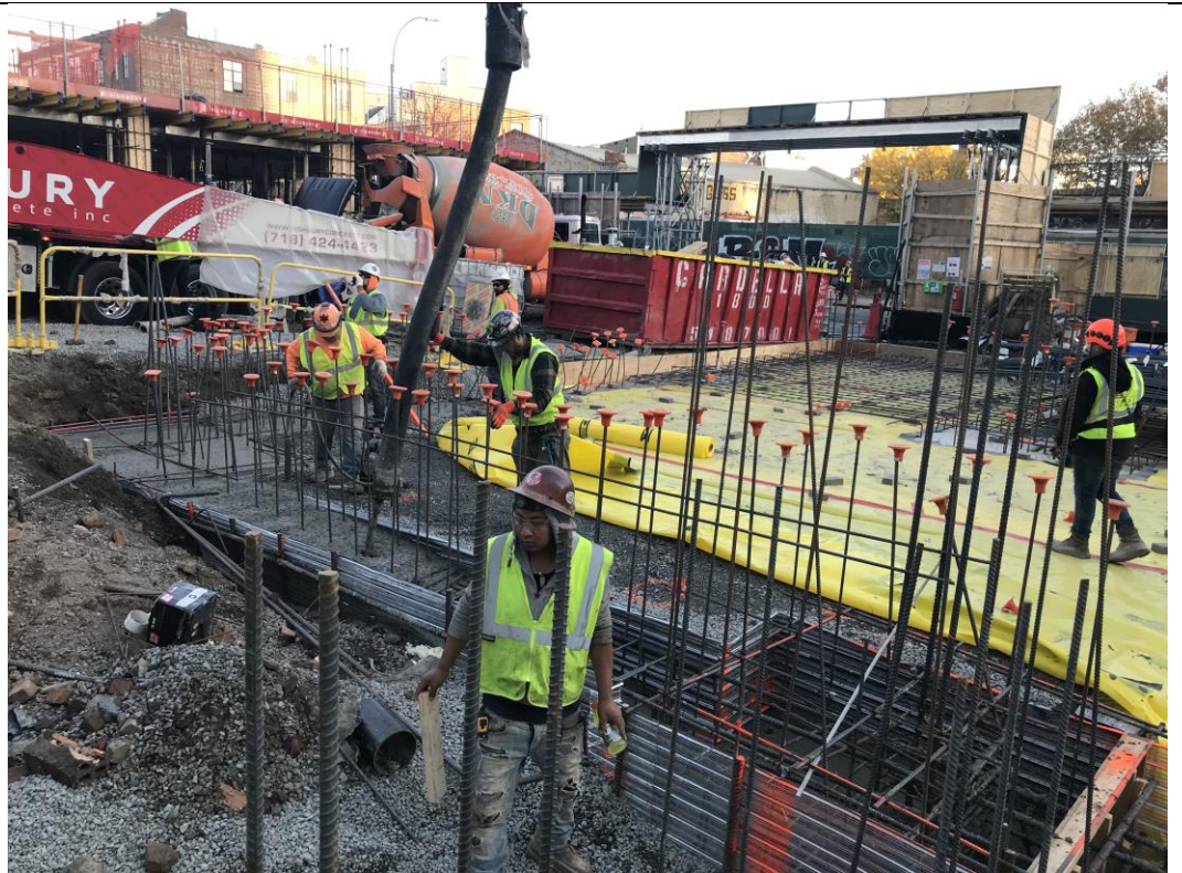
Photo 2: View of STNY pouring concrete into pile cap and grade beam formwork in waste characterization grid COMP H (facing southeast).
