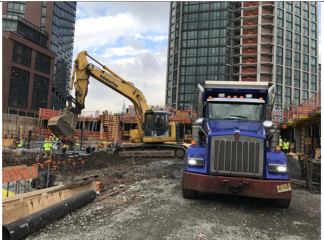
Photo 2: View of STNY loading a truck with soil for off-site disposal to the CEPA facility (facing north).
