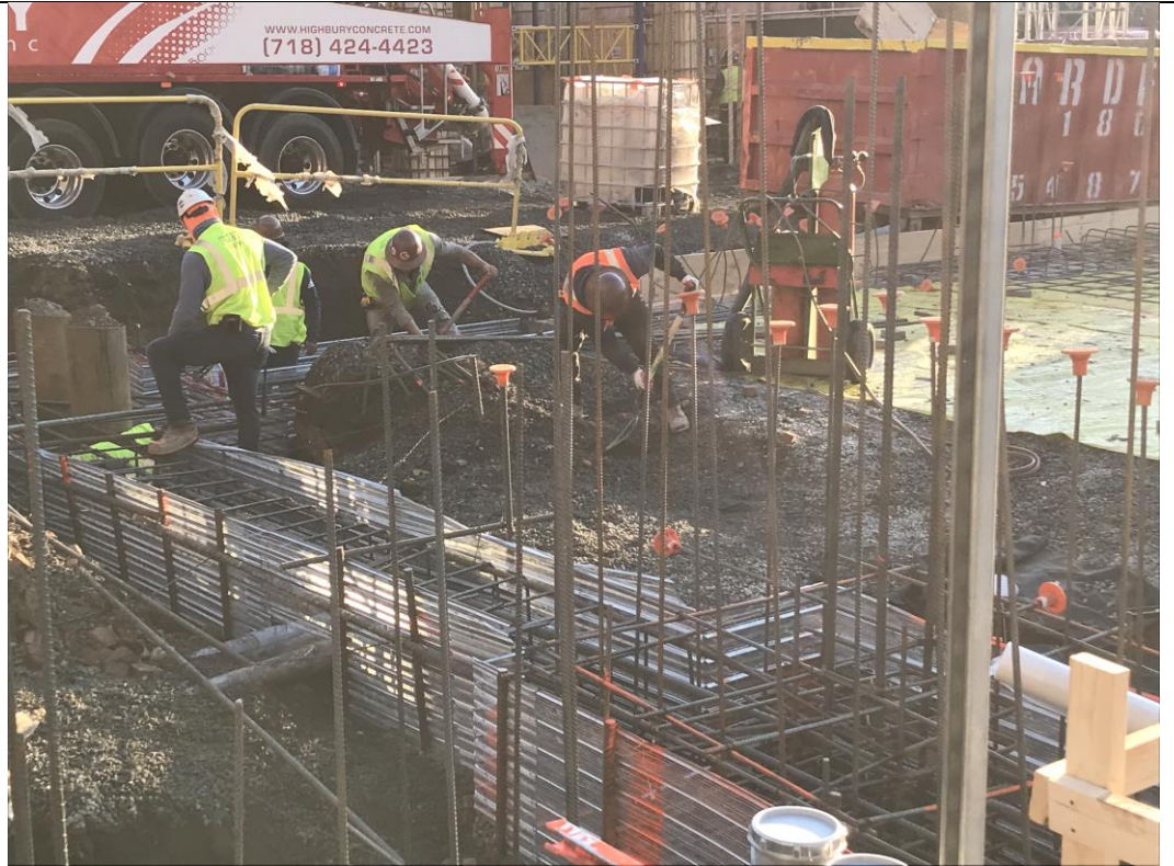
Photo 1: View of STNY installing pile cap and grade beam formwork in waste characterization grid COMP H (facing southeast).
