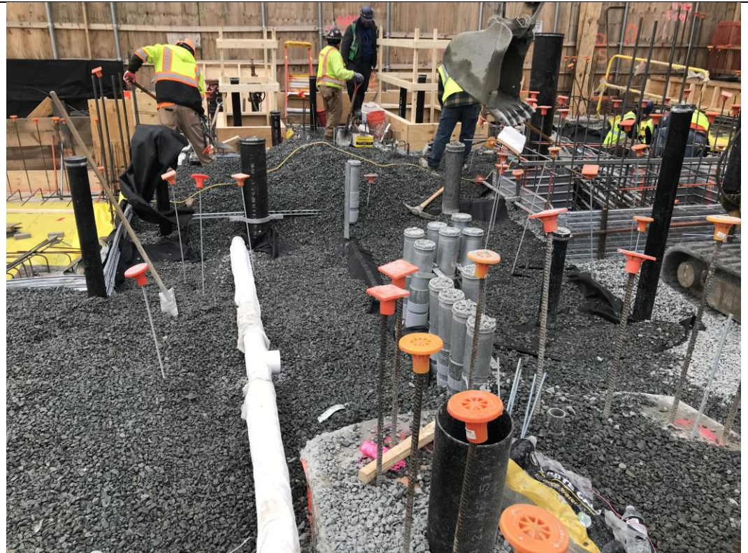
Photo 2: View of STNY installing SMD system components in waste characterization grid COMP G (facing west).
