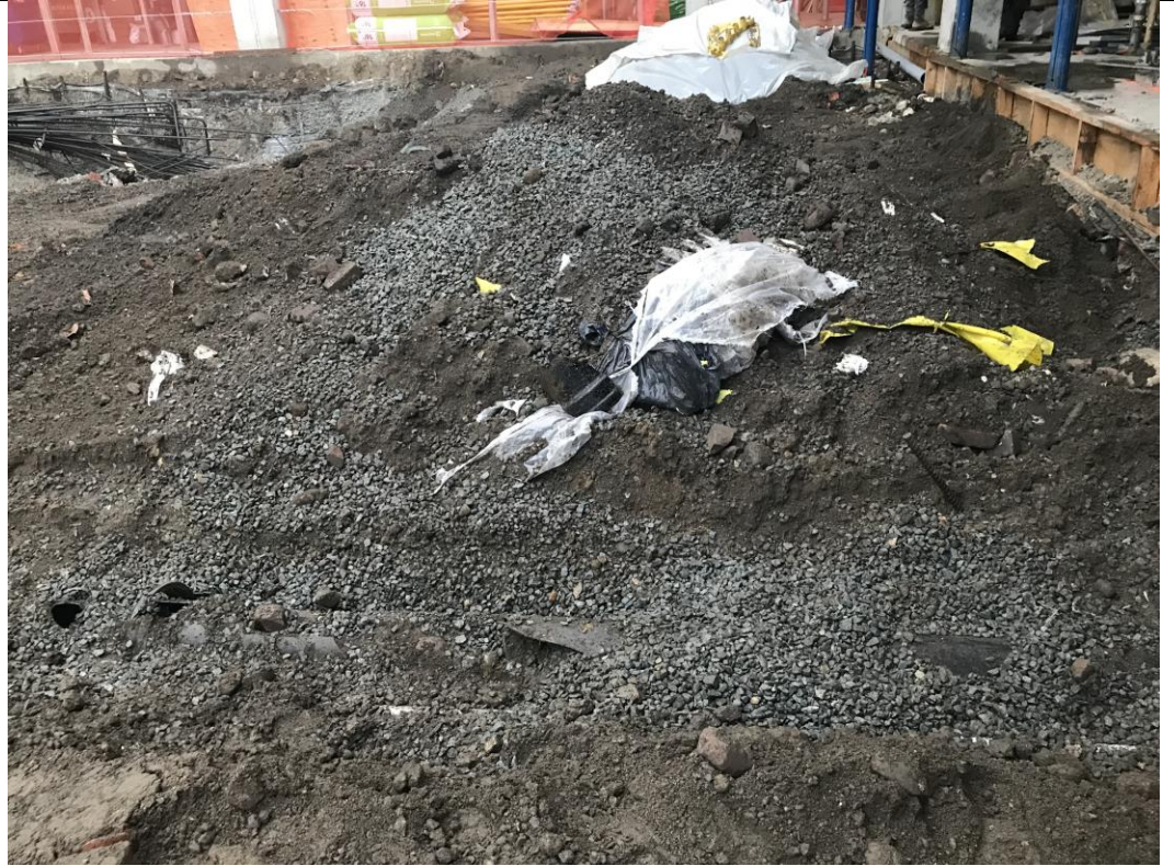
Photo 3: View of utility repair excavation in waste characterization grid COMP J South (facing north).
