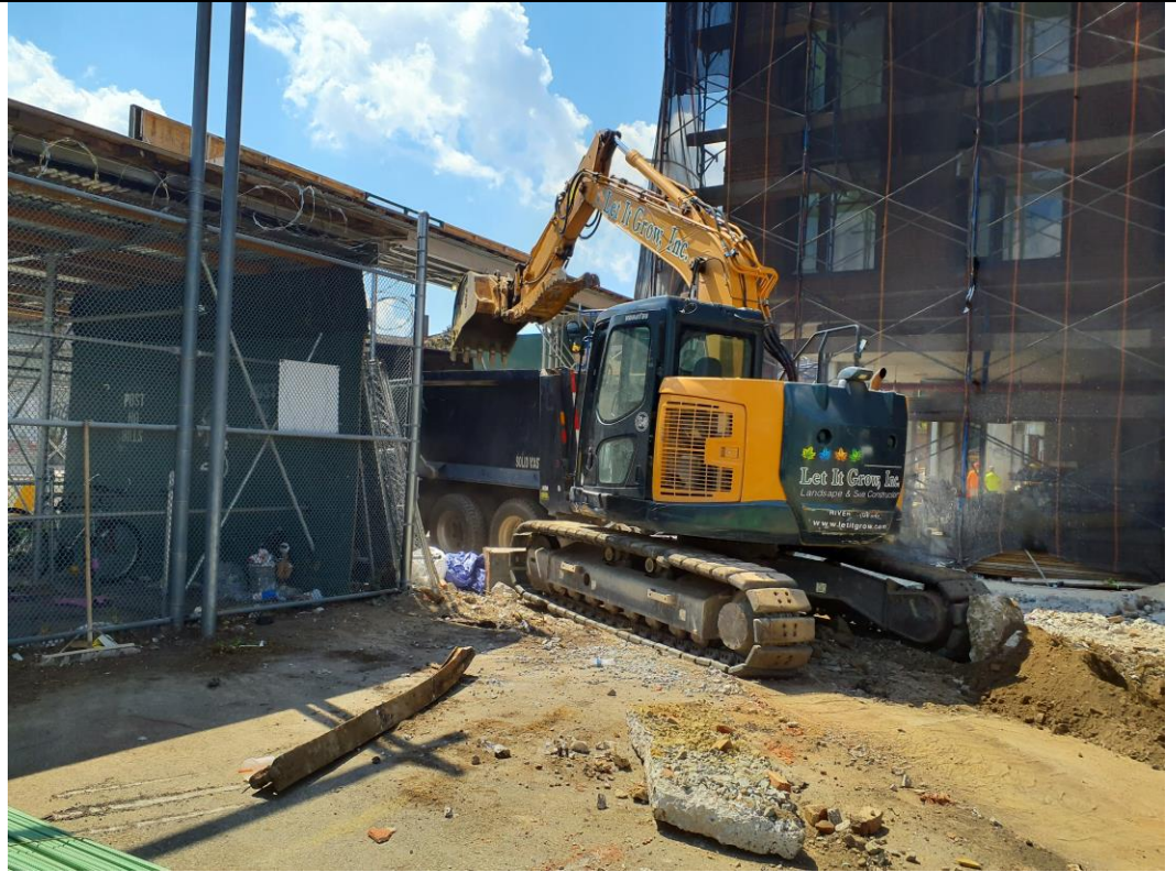
Photo 3: View of Let It Grow loading a truck for off-site disposal to the CEC facility (facing southwest).
