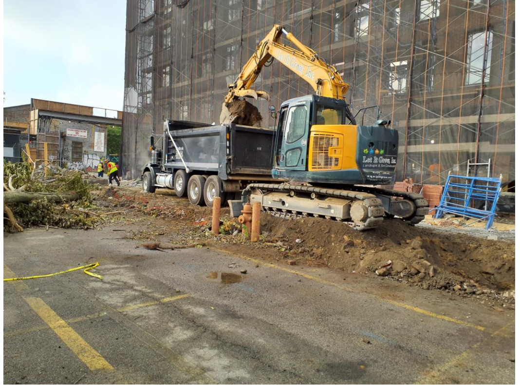
Photo 3: View of Let It Grow loading a truck for off-site disposal to the CEC facility (facing southwest).
