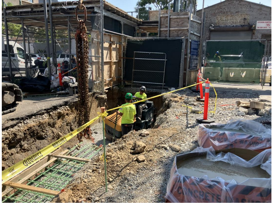
Photo 3: View of Let It Grow compacting the 0.75-inch stone backfill (facing south).
