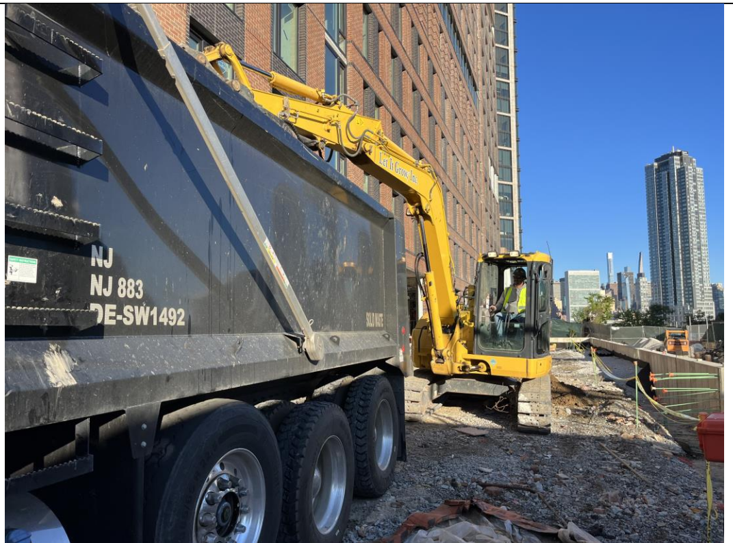
Photo 2: View of Let It Grow loading a truck with excavated soil for off-site disposal to the CEC facility (facing north).
