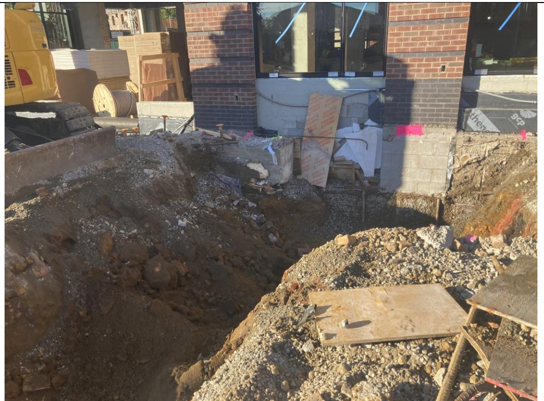
Photo 2: View of Let It Grow excavating in waste characterization grid COMP K for a retaining wall (facing west).
