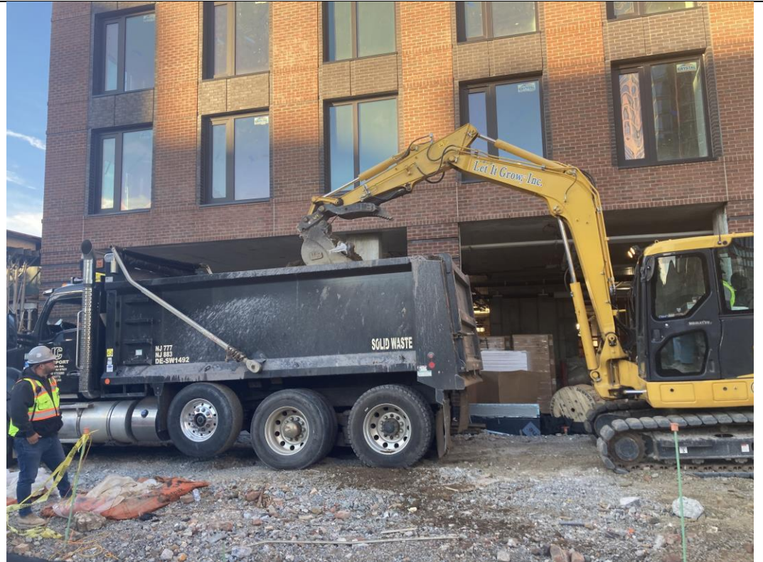
Photo 1: View of Let It Grow loading a truck with excavated soil for off-site disposal to the CEC facility (facing west).
