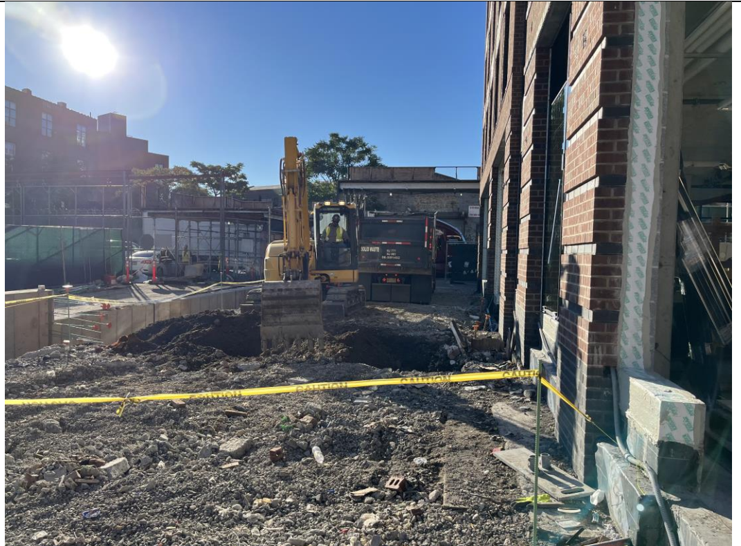
Photo 1: View of Let It Grow excavating in waste characterization grid COMP K for the retaining wall (facing south).
