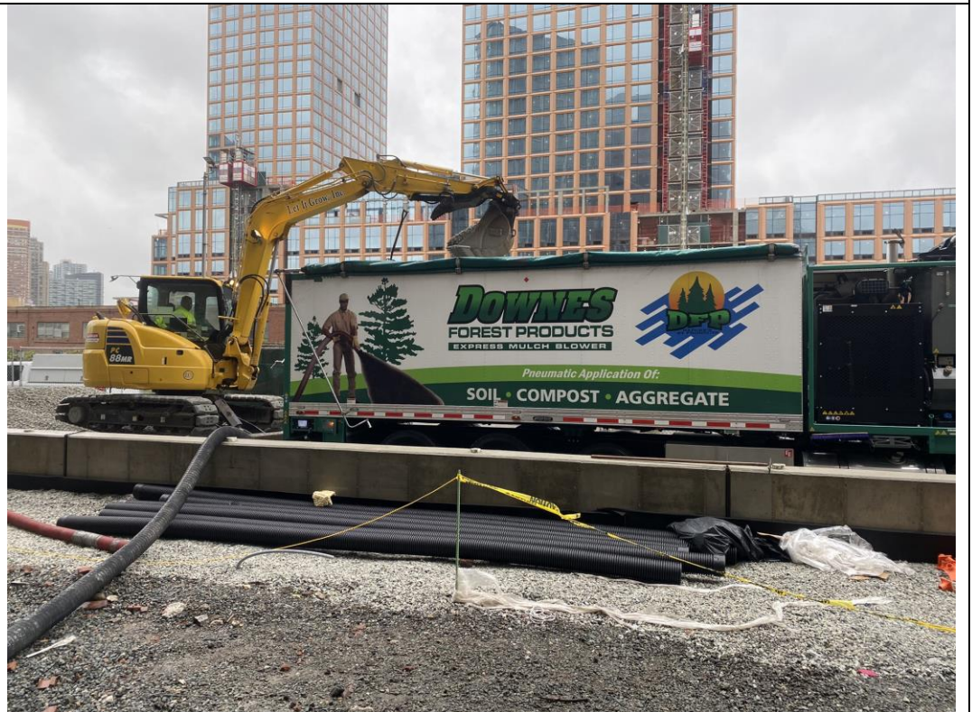
Photo 2: View of Let It Grow loading 0.75-inch stone into the pneumatic blower to backfill the north courtyard (facing northeast).
