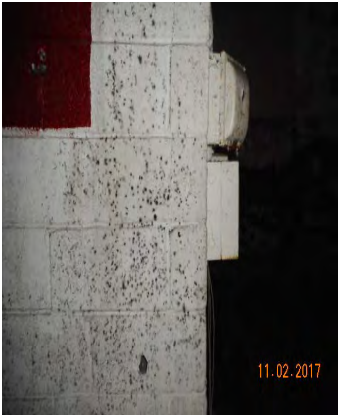
First floor- visible mold growth
