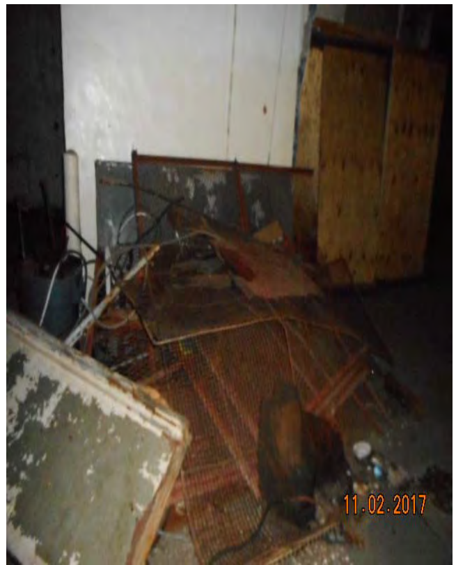
First floor-building debris
