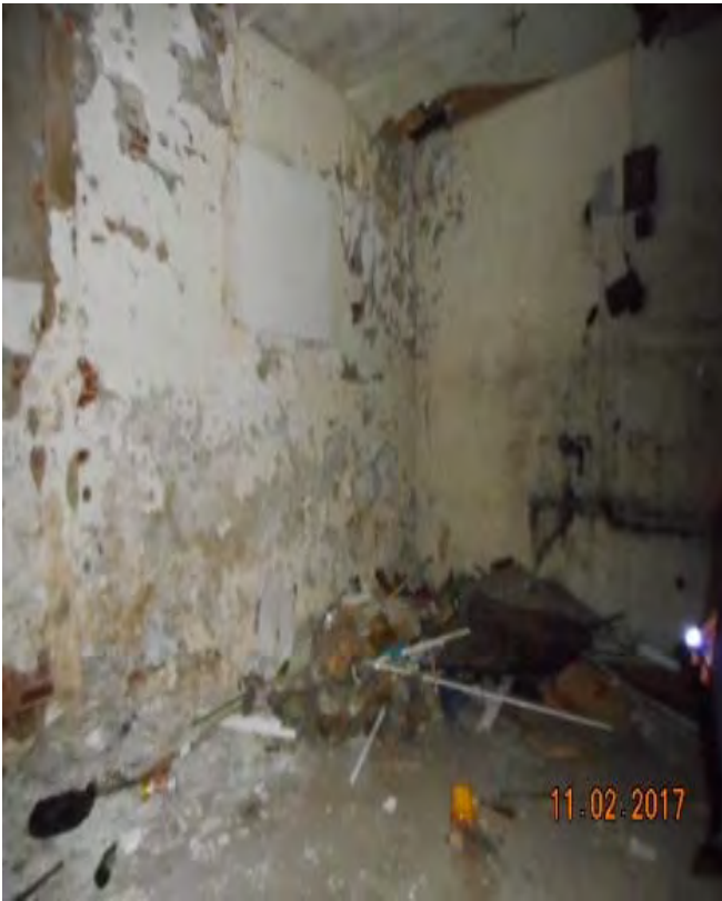
First floor-building debris
