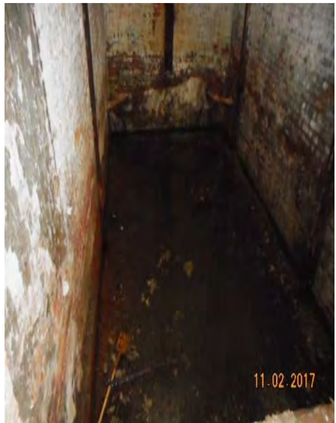
First floor- standing water in the empty elevator shaft
