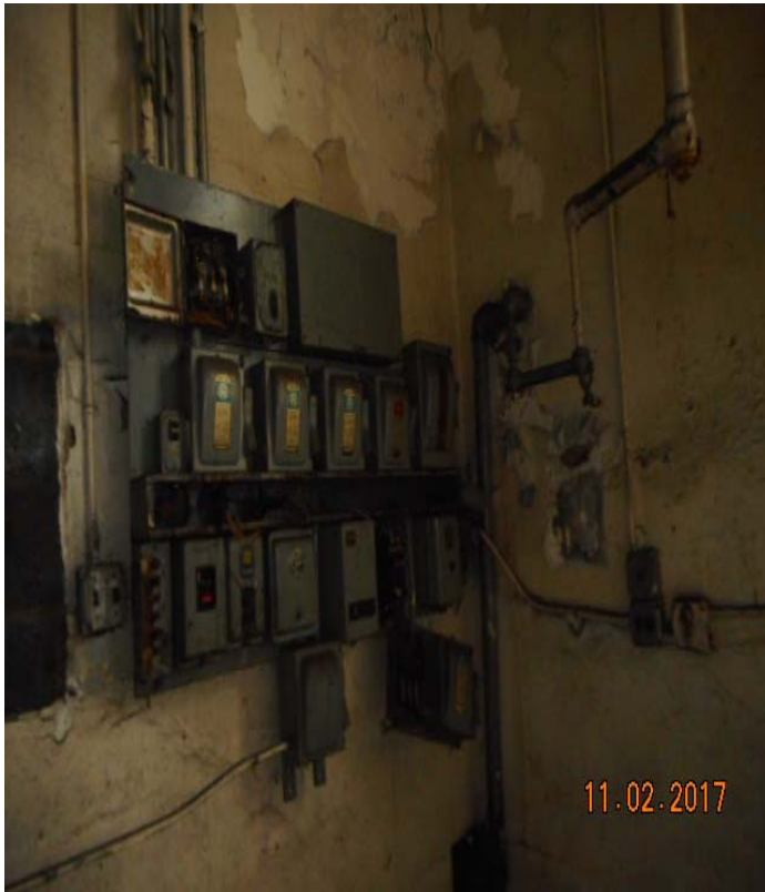
First floor- electrical panels
