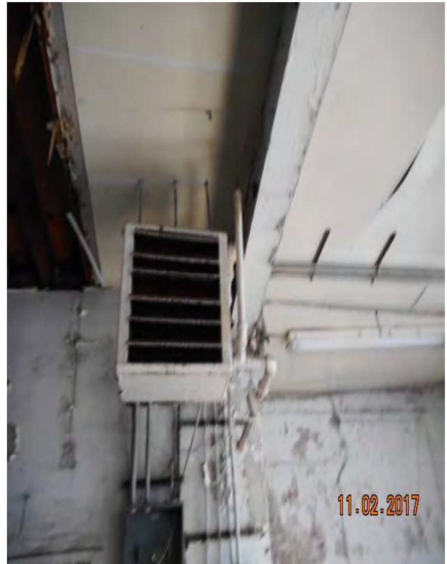
Second floor- typical space heater
