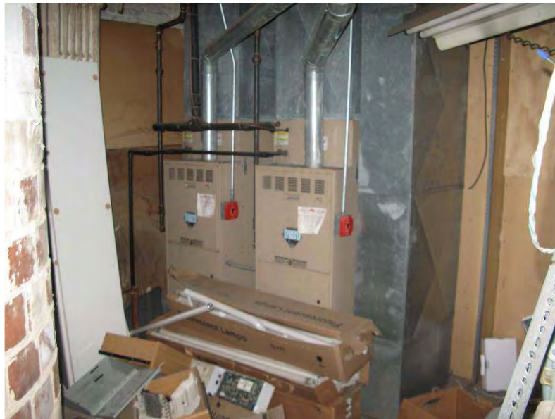
Photo 19: Mechanical room at 473-491 President Street.
