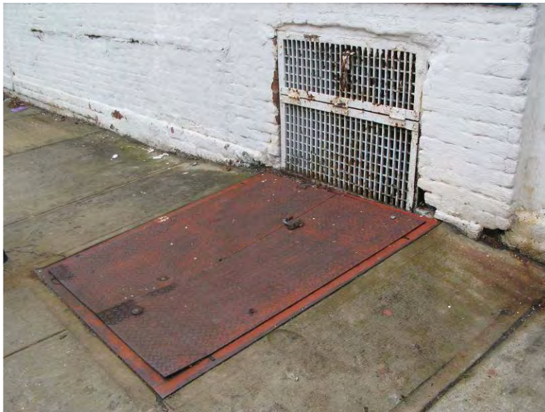
Photo 15: Storage tank vault area outside the President Street building.
