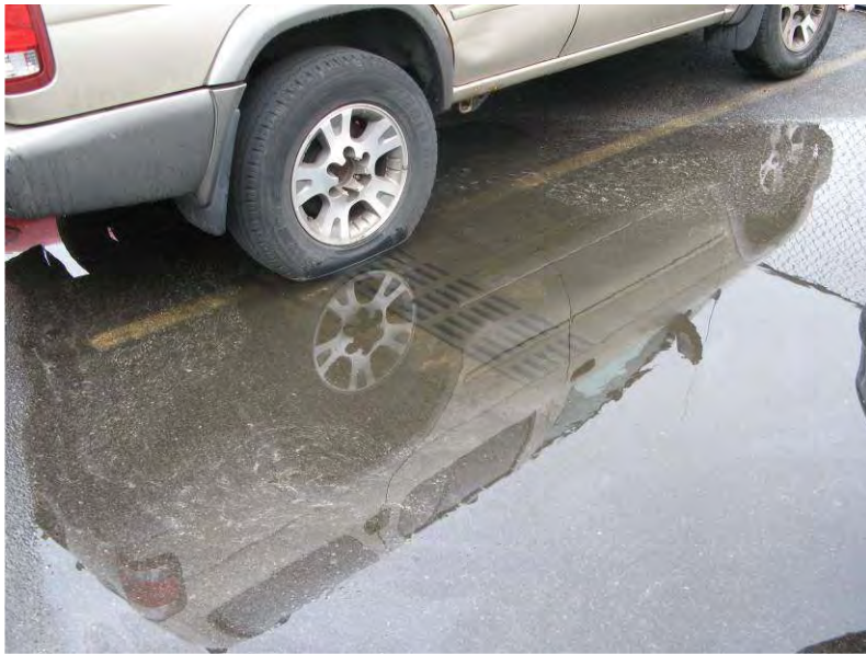
Photo 3: Drain inlet with ponded water on the Nevins Street/Carroll Street lot.
