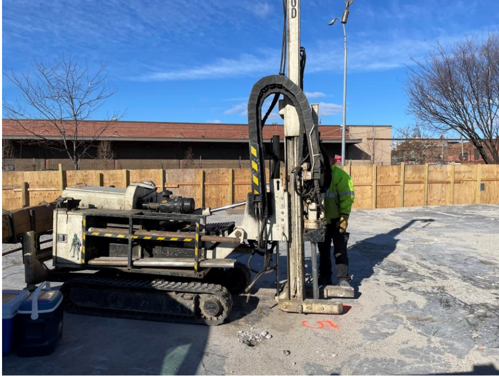
Photo 1: Lakewood advancing soil boring EB05 in the western part of the site (facing west)
