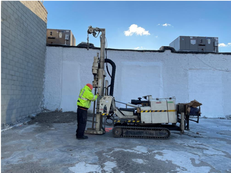
Photo 2: Lakewood advancing soil boring EB02 in the western part of the site (facing east)
