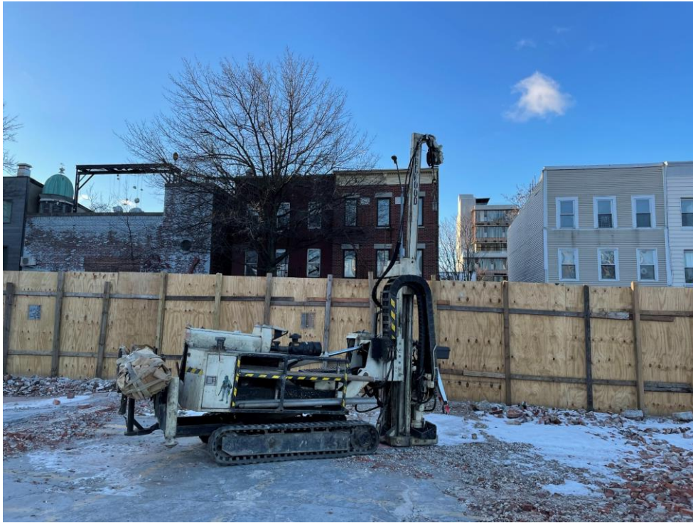
Photo 1: Lakewood advancing soil boring EB15 in the southeastern part of the site (facing south)
