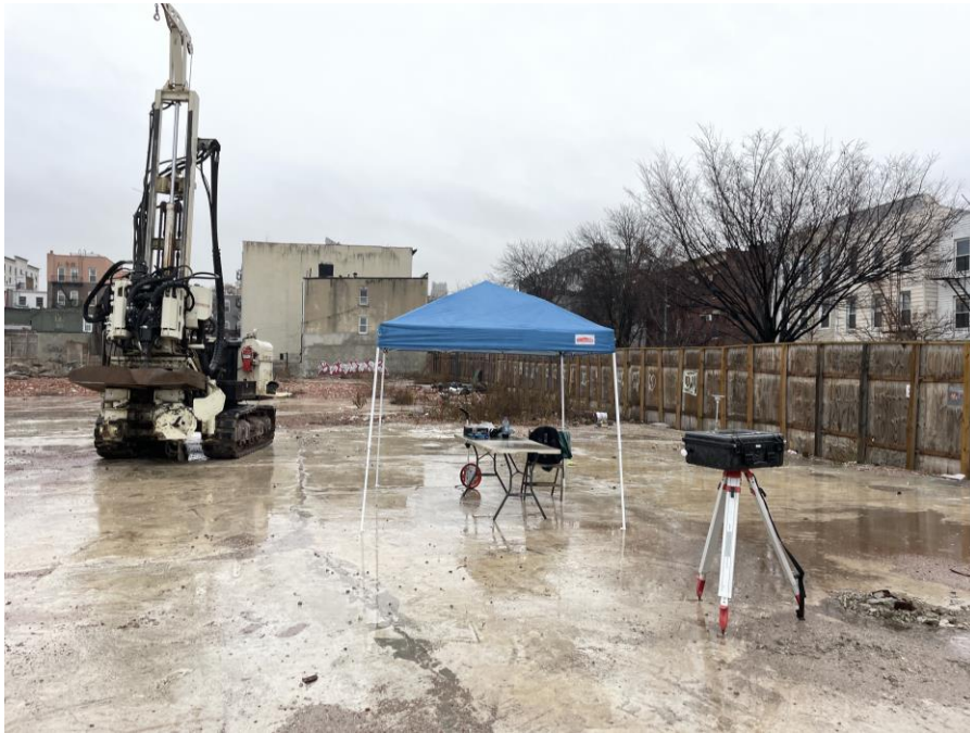
Photo 1: Eastern Environmental advancing soil boring SB03_CT in the central part of 473 President Street (facing southeast)
