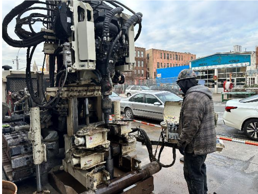
Photo 1: Eastern Environmental advancing soil boring SB01_CT on the Union Street sidewalk (facing north)
