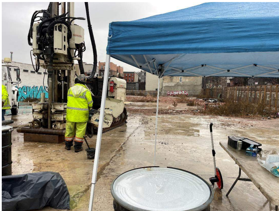
Photo 8: Eastern advancing soil boring SB03_CT near MW-20D on the 473 President Street site (facing east) 12/22/2022
