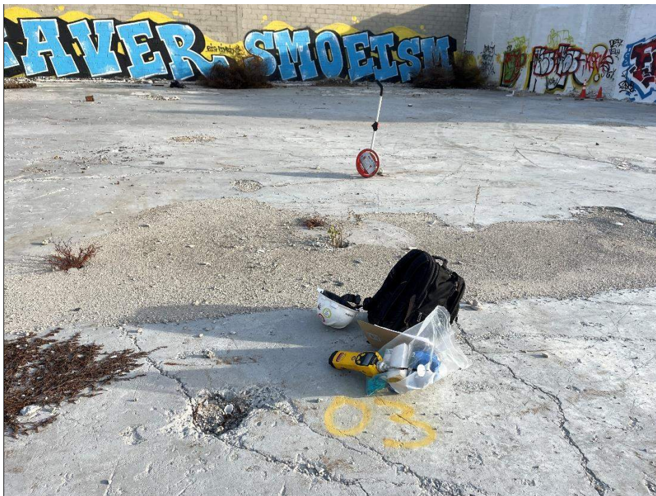
Photo 1: Soil Boring SB02_CT marked out near MW-03 on the E-Waste Parcel site (facing northeast) 12/21/2022
